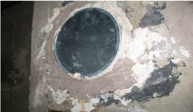
Photo 2: View of asbestos-containing boiler insulation associated with the chimney observed in Room 002 in the basement of the subject building.
