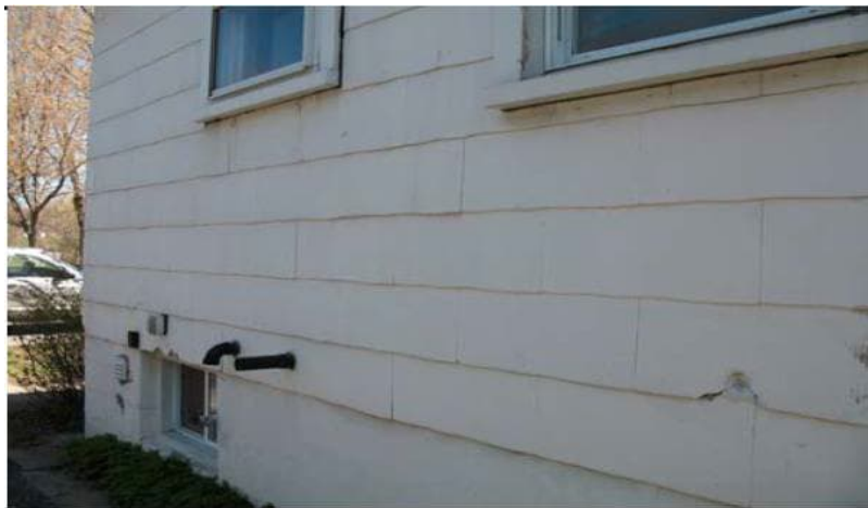
Photo 4: View of asbestos-containing siding-transite observed on the exterior of the subject building.
