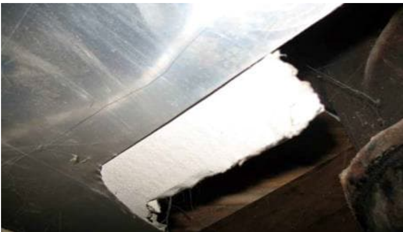
Photo 3: View of asbestos-containing aircell pipe insulation observed in Room 002 in the basement of the subject building.
