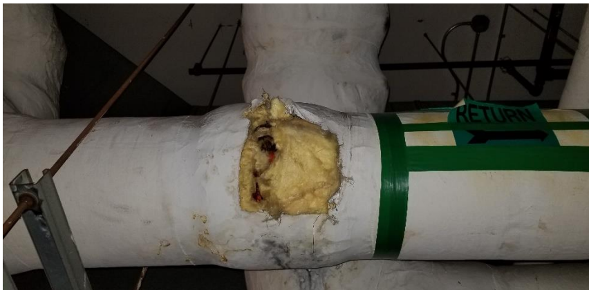
Photo 2: Representative view of the non-asbestos-containing mechanical insulation observed throughout the subject building.
