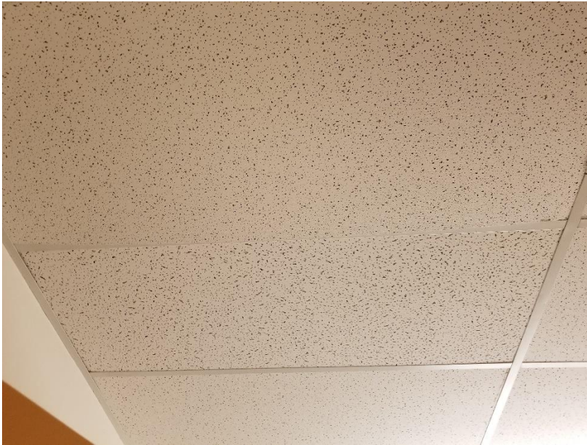
Photo 3: View of non-asbestos-containing suspended ceiling tiles (Pinholes w/ Large Fissure).
