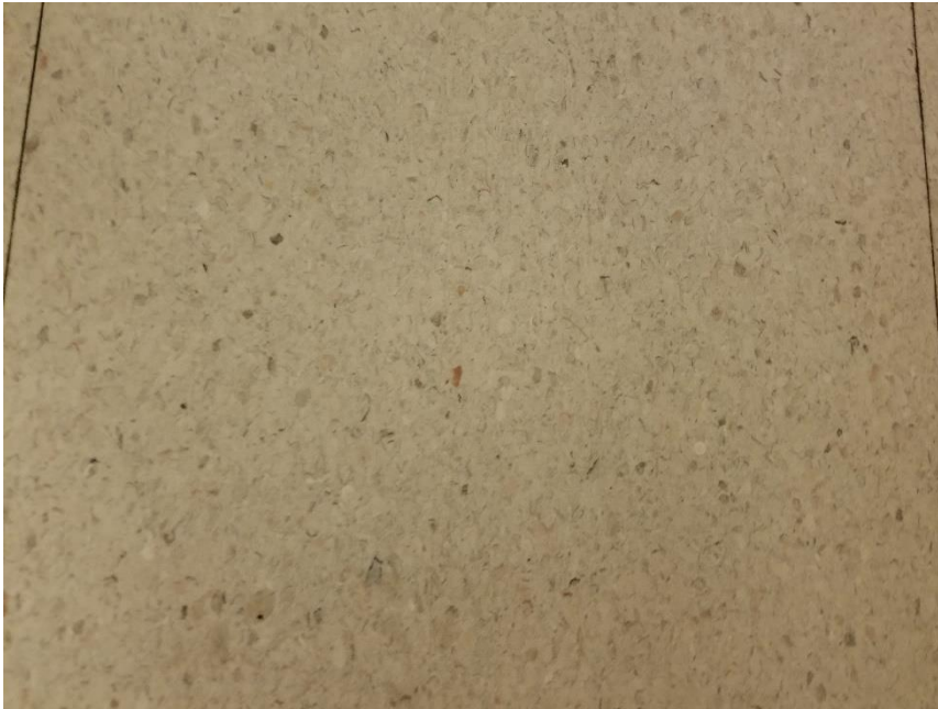
Photo 5: View on non-asbestos containing vinyl floor tiles (12"x12"- White, Brown & Grey Flakes)
