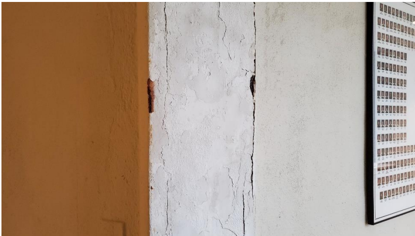
Photo 5: View of the non-asbestos containing wall plaster observed throughout the subject building.
