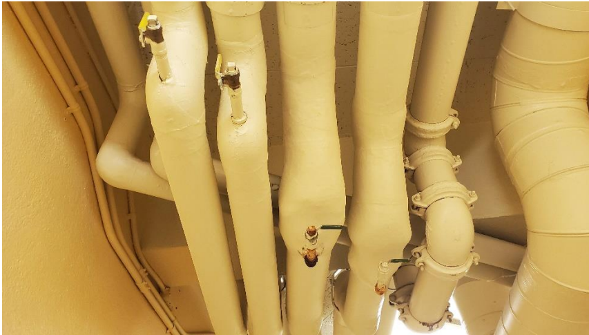
Photo 4: View of the asbestos-containing parging cement pipe elbow/fitting insulation observed in good condition in Room 014B.
