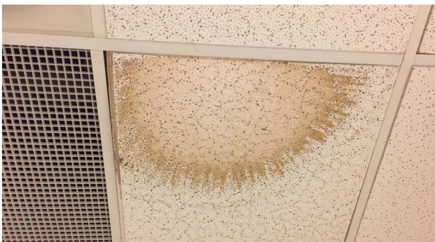
Photo 12: View of the water damaged ceiling tiles observed in Room 0011A.
