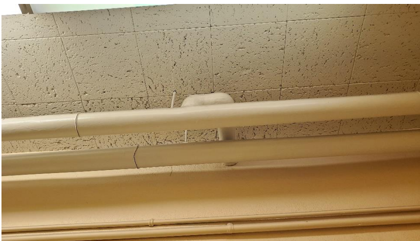
Photo 6: Representative view of the asbestos containing ceiling tiles (1'x1' – Pinholes and Large Fissures) observed in good condition.
