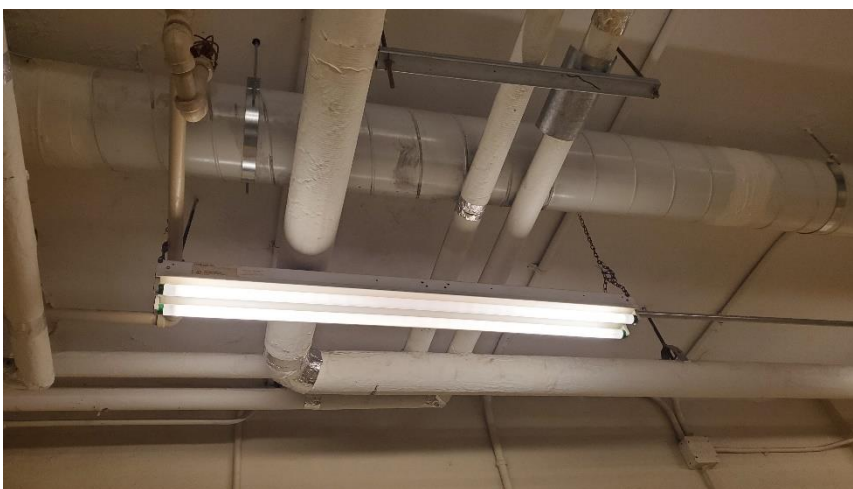
Photo 3: Representative view of the fluorescent light fixtures containing mercury vapour, observed throughout the subject building.
