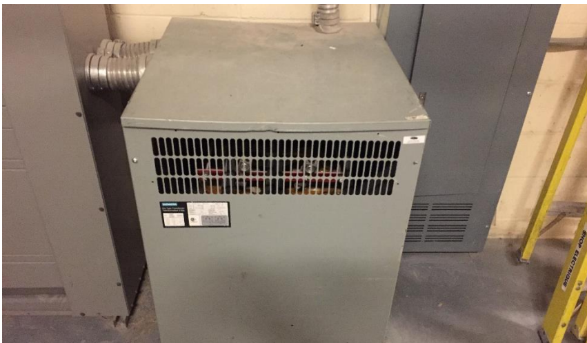
Photo 8: View of the non-PCB dry-type transformers observed throughout the subject building.
