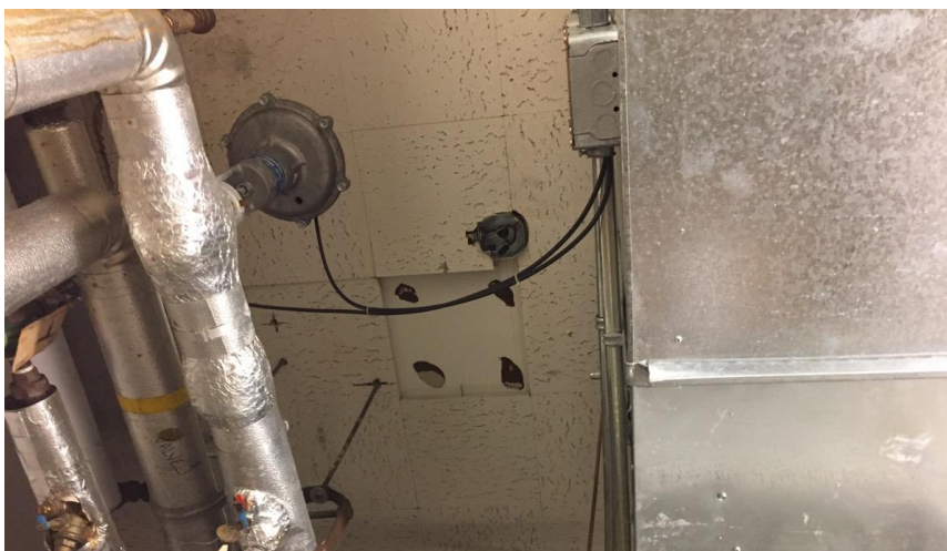
Photo 11: Representative view of the asbestos containing ceiling tiles (1'x1' – Pinholes and Large Fissures) observed in Room 023A.
