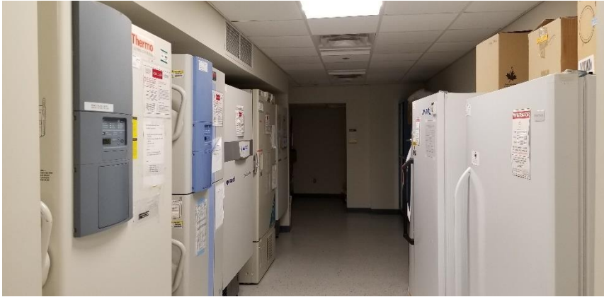
Photo 31: Representative view of the equipment observed throughout the third floor, containing ozone depleting substances.
