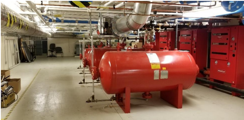
Photo 2: Representative view of the above ground foam tanks observed in Room 0507.
