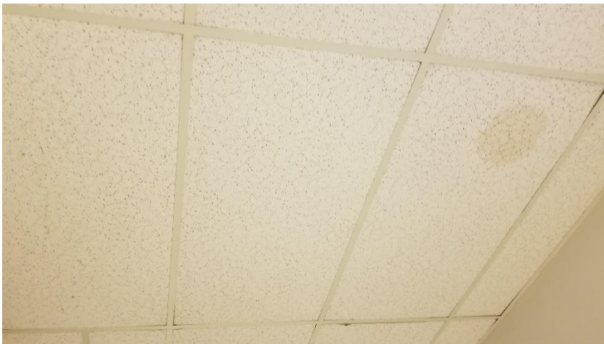
Photo 26: Representative view of water damaged ceiling tiles observed throughout the subject building.
