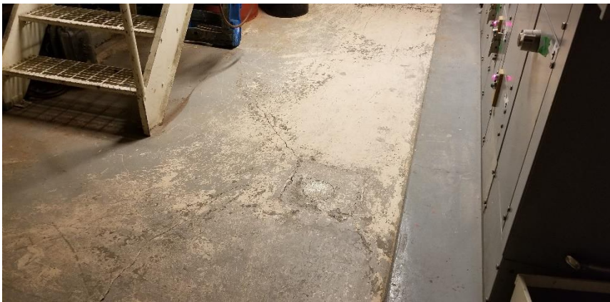
Photo 5: View of the poor condition lead floor paint (Grey) observed in Room 1138.
