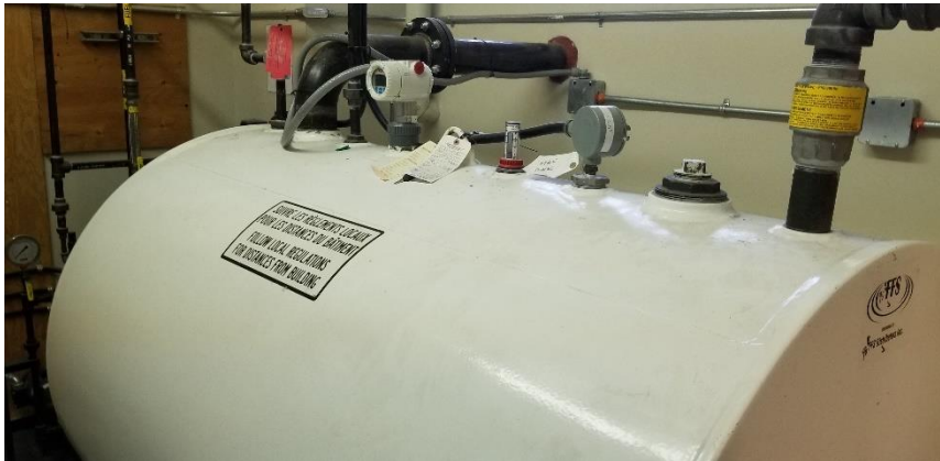
Photo 7: View of the above ground diesel storage tank observed in Room 1129C.
