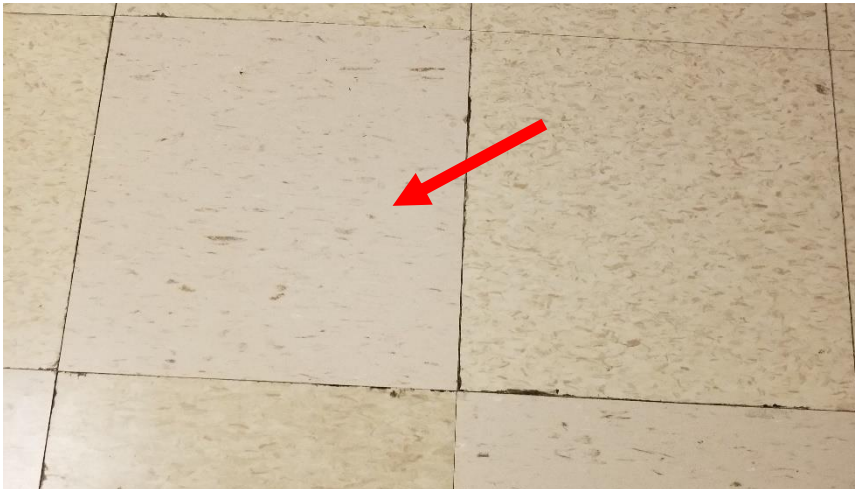
Photo 11: Representative view of the asbestos containing VFT (12"x12" Beige w/ Grey Flakes) observed throughout the subject building.
