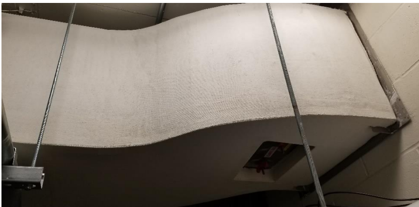
Photo 3: Representative view of the fiberglass insulation observed on HVAC ducts in Room 0515.
