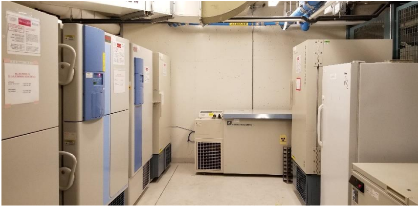
Photo 1: Representative view of refrigeration equipment observed in Room 0509, containing various ozone depleting substances.
