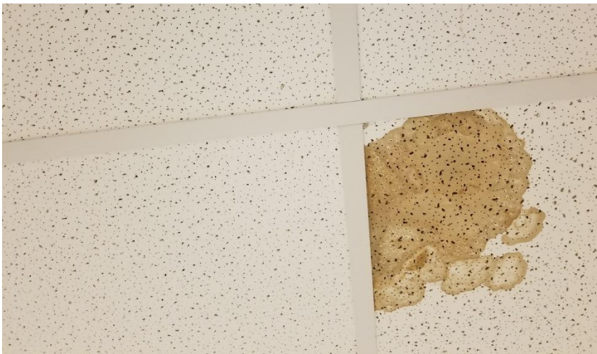
Photo 35: Representative view of water damaged ceiling tiles observed throughout the subject building.
