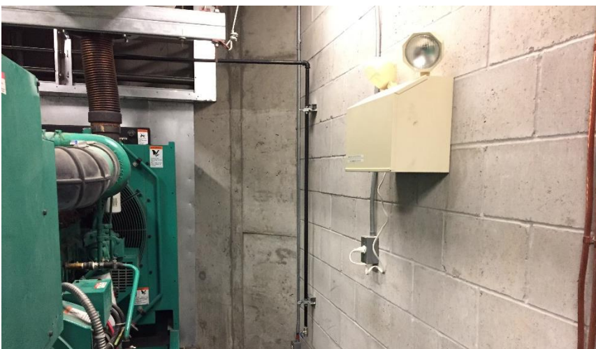
Photo 9: View of the lead-containing battery pack observed in Room 0005.
