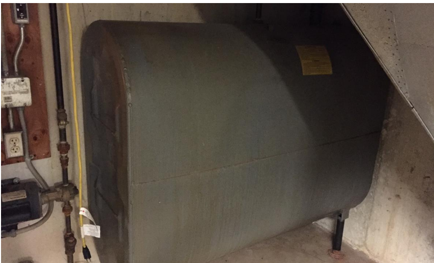
Photo 6: View of the above-ground storage tank containing diesel fuel in Room 0004.
