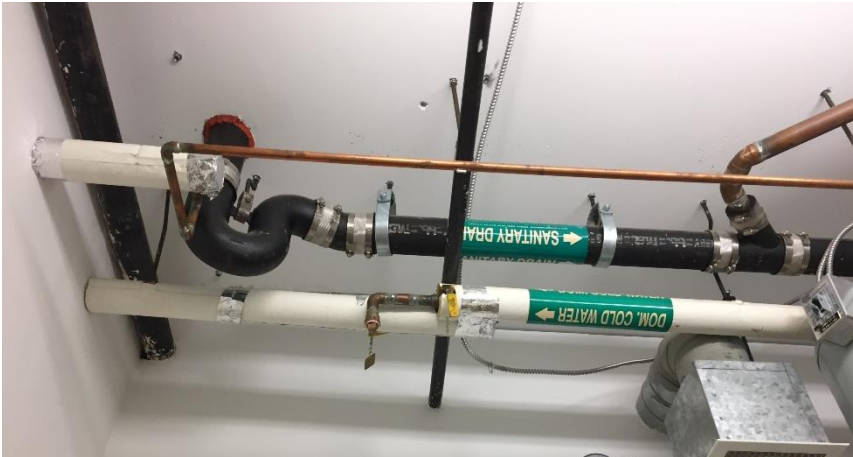
Photo 4: Representative view of the non-asbestos-containing mechanical insulation observed throughout the subject building.
