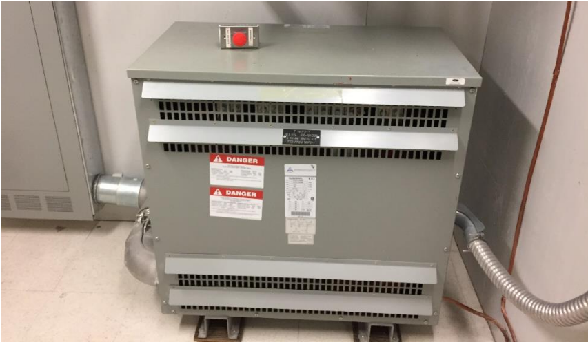
Photo 7: Representative view of the non-PCB containing dry-type transformers observed throughout the subject building.
