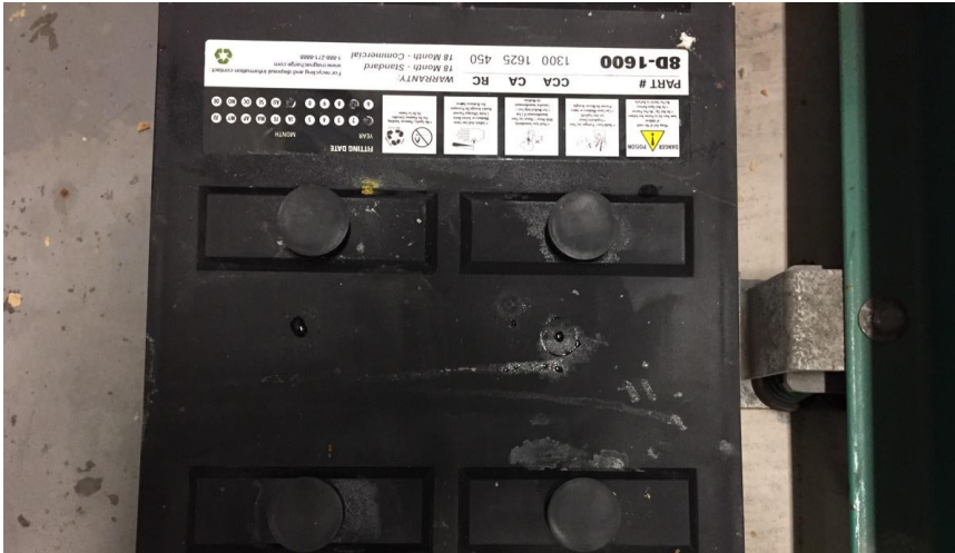
Photo 10: View of the lead-containing battery pack observed in Room 0005.
