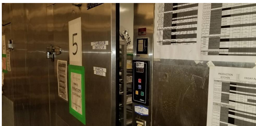
Photo 23: View of Foster walk-in freezer containing R-12 refrigerant in area 0044.
