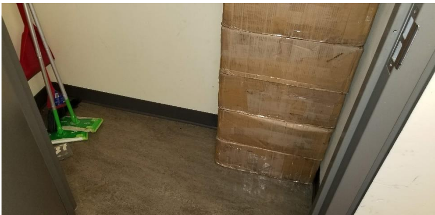
Photo 15: View of non-asbestos containing vinyl sheet flooring (Gray) observed in Room 031C.
