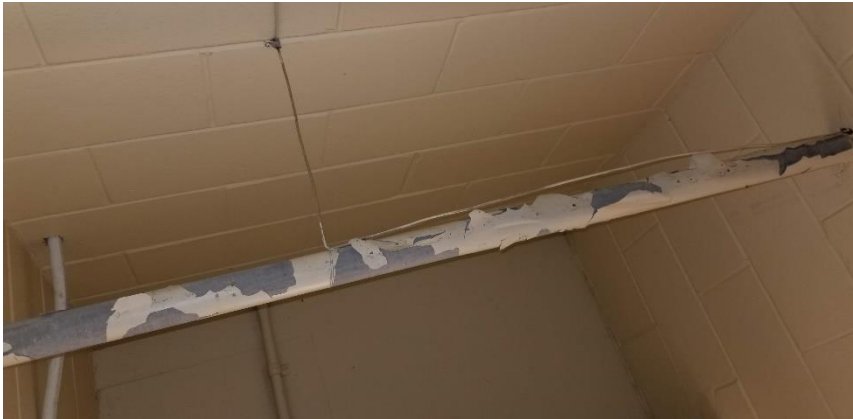
Photo 19: View of lead paint finish (Off-White) observed to be in poor condition on a mechanical pipe in Room 017.
