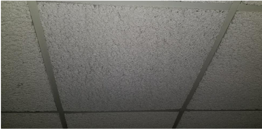
Photo 16: View of non-asbestos containing suspended ceiling tiles (2'x2'-Deep Texture) observed in 014 Hallway.
