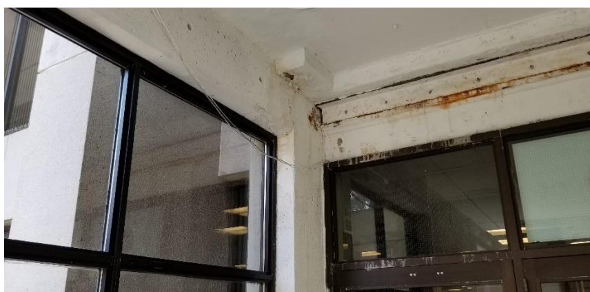
Photo 24: View of water staining observed on concrete ceiling deck and walls in the 022B Hallway.
