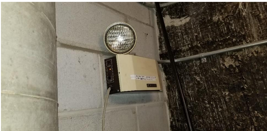
Photo 21: View of lead containing battery packs observed in Room 0033A.
