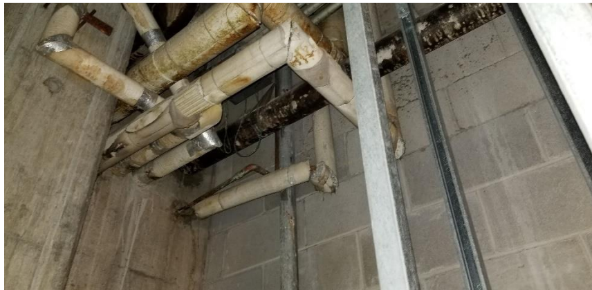
Photo 7: View of asbestos-containing mechanical pipe straight insulation (AirCell) observed to be in poor condition in Room 0033B.
