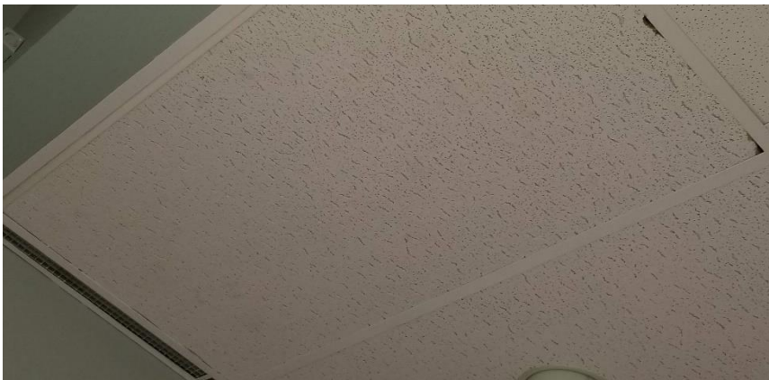
Photo 17: View of non-asbestos containing suspended ceiling tiles (2'x4'-Pinholes with Large Fissures) observed in Room 211.
