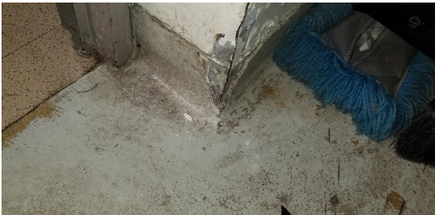
Photo 11: View of asbestos-containing cementitious floor coating observed in Room 210.
