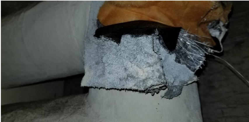
Photo 4: View of asbestos-containing parging on pipe fitting observed in Room 100G.
