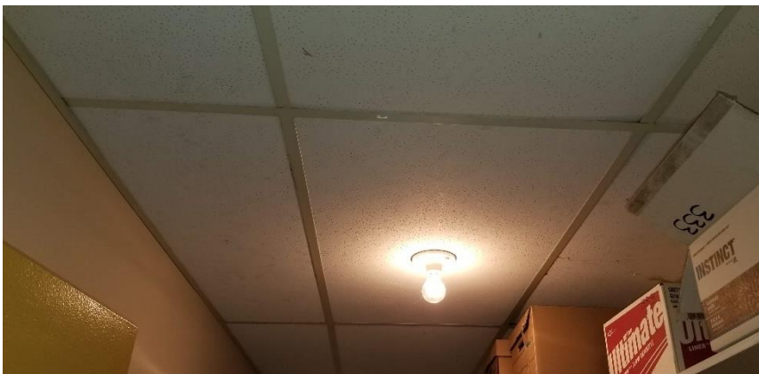
Photo 12: View of asbestos-containing suspended ceiling tiles (2'x4'-White with dots) observed to be in Room 333B.
