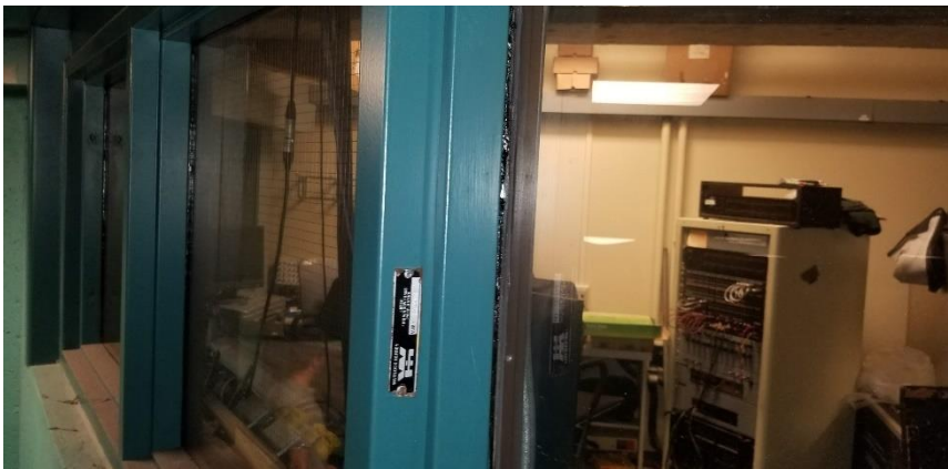
Photo 2: View of asbestos-containing window caulking (Black) observed to be in good condition outside of Room 100G.
