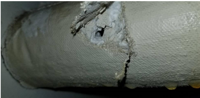
Photo 5: View of asbestos-containing parging observe in pipe straight in Room 0029.
