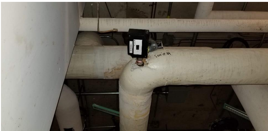
Photo 6: View of asbestos-containing parging cement on pipe fitting observed to be in poor condition in Room 0033H.
