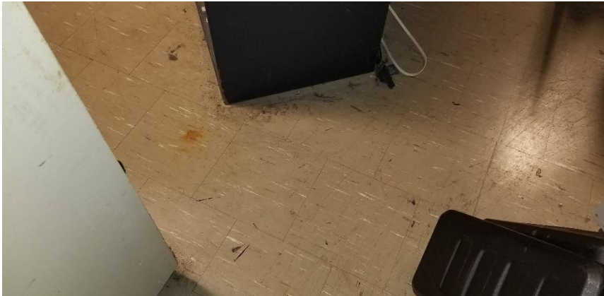
Photo 1: View of asbestos-containing vinyl floor tiles (12"x12"-Beige with White and Brown Flakes) observed to be in good condition in Room 100G.
