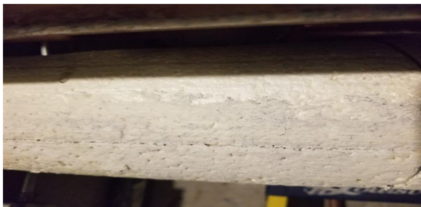
Photo 8: View of asbestos-containing parging on foam pipe insulation observed to be in good condition in Room 0027.
