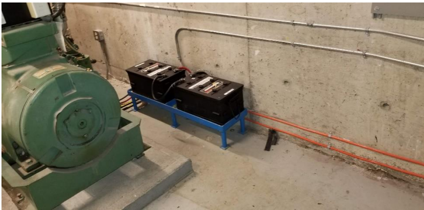
Photo 20: View of lead containing acid batteries observed to be in good condition in Room 0033H.
