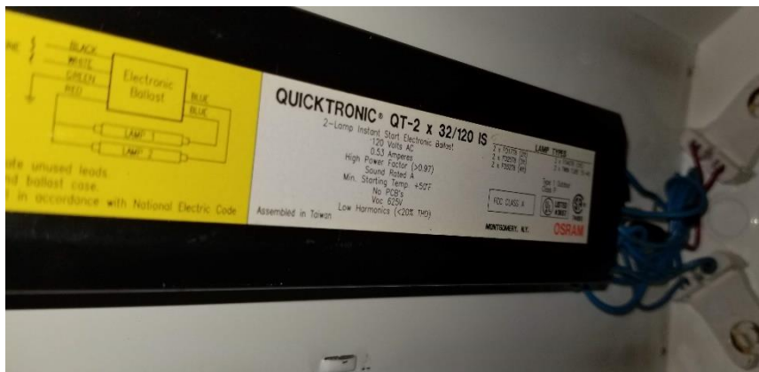
Photo 22: View of non-PCB containing light ballast observed in Room 100G.
