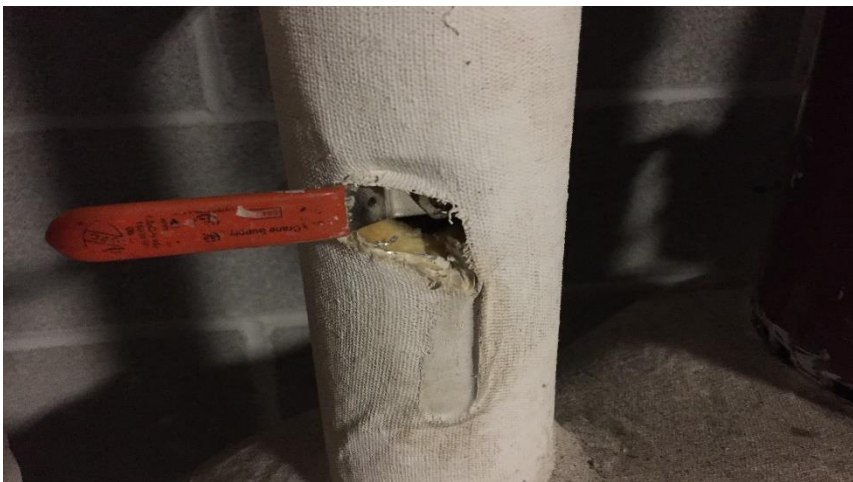
Photo 5: Typical view of fibreglass mechanical insulation.
