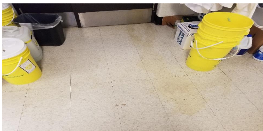
Photo 12: View of non-asbestos containing vinyl floor tiles (12"x12"-White with Grey Flakes) observed in Room D511.
