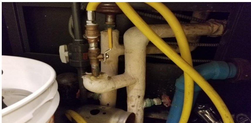
Photo 1: View of asbestos-containing parging cement on fitting observed to be in fair condition underneath the sink in D320.
