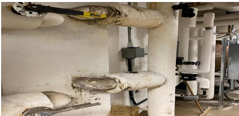
Photo 7: View of mould/water damaged mechanical pipe straights observed in E101.
