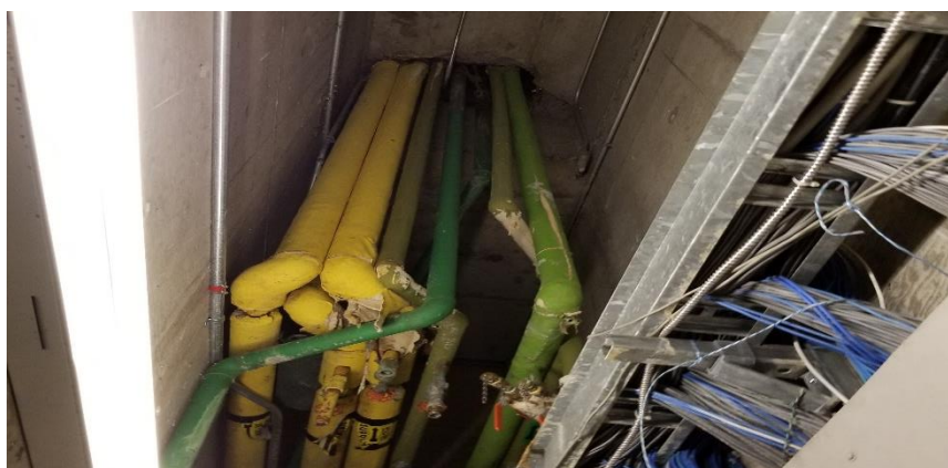
Photo 2: View of asbestos-containing parging cement on fittings observed to be in poor condition in Room C012B.
