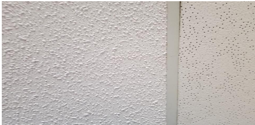
Photo 10: View of non-asbestos ceiling tiles: Pinholes with texture (left) and Pinholes with varying sizes (right) observed in B109C.
