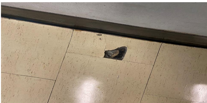
Photo 9: View of fair condition ACM Vinyl Floor Tile (12"x12"-White with Grey Flakes) observed in Location A710.
