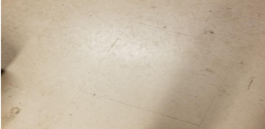
Photo 13: View of non-asbestos containing vinyl floor tiles (12"x12"-Grey ) observed in Room E018B.
