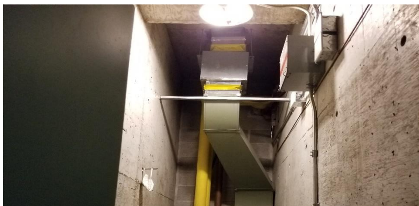
Photo 11: View of non-asbestos containing flexible duct connector observed in Room C503.
