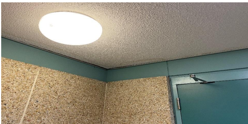
Photo 8: View of poor condition presumed asbestos ceiling texture finish observed in the Hallways outside of A502.
