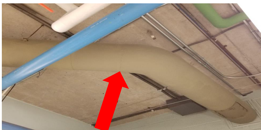
Photo 5: View of asbestos-containing duct insulation observed to be in good condition in Room D320.
