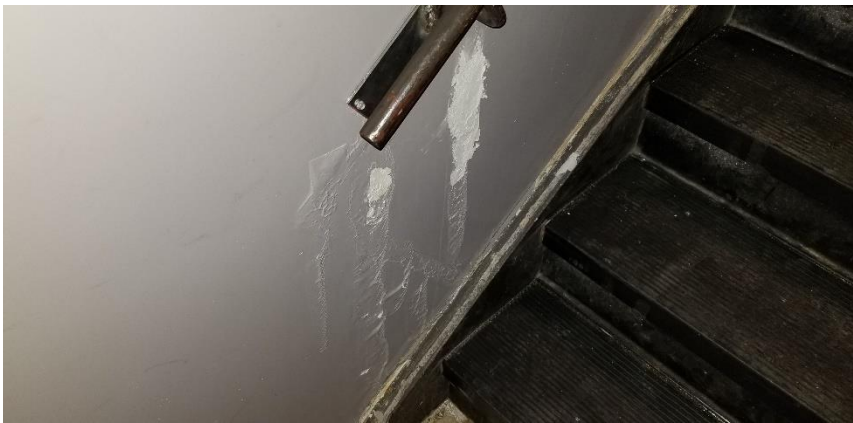
Photo 5: View of the water damaged drywall observed in Room 600.
