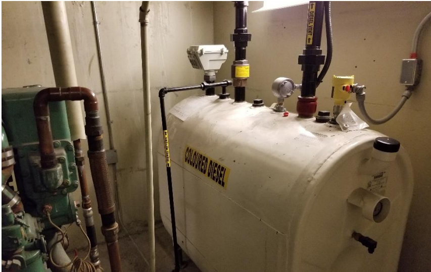
Photo 27: View of the above ground storage tank (AST) containing diesel, observed in good condition in Room 142C.
