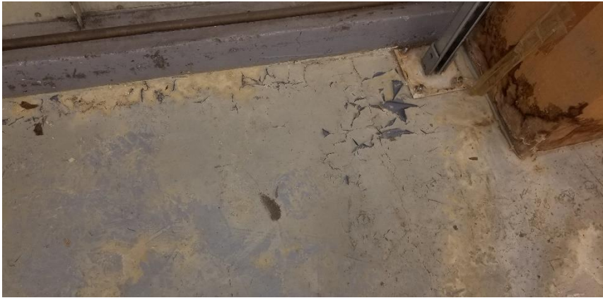
Photo 4: View of the poor condition lead floor paint (Grey) observed throughout Room 600.
