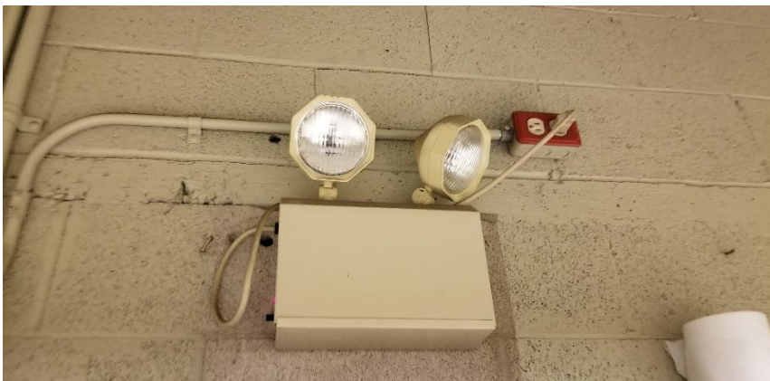
Photo 3: View of the lead battery packs associated with emergency lighting observed in Room 600.
