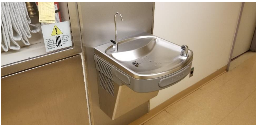
Photo 12: Representative view of the water fountains observed throughout the subject building, containing ODSs.
