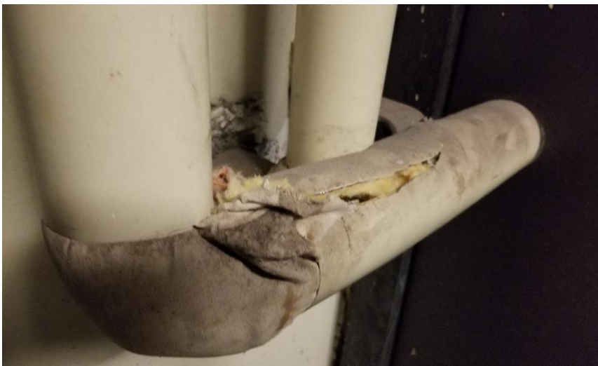
Photo 18: View of the non-asbestos fiberglass pipe straight insulation observed in Room 348.
