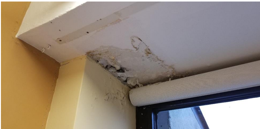
Photo 11: View of the water damaged drywall observed in Room 528.
