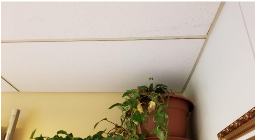
Photo 20: View of the asbestos containing ceiling tiles - 2'x4' Pinholes w/ Triangular Fissures observed in good condition in Room 306.
