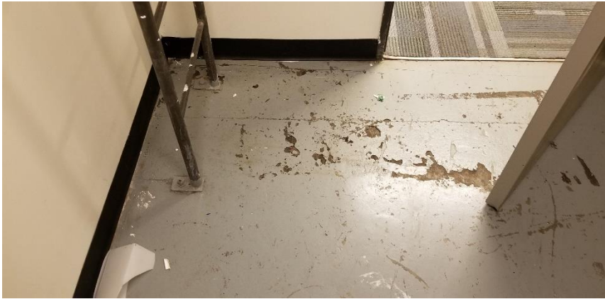
Photo 10: View of the poor condition lead floor paint (Grey) observed throughout Room 525E.
