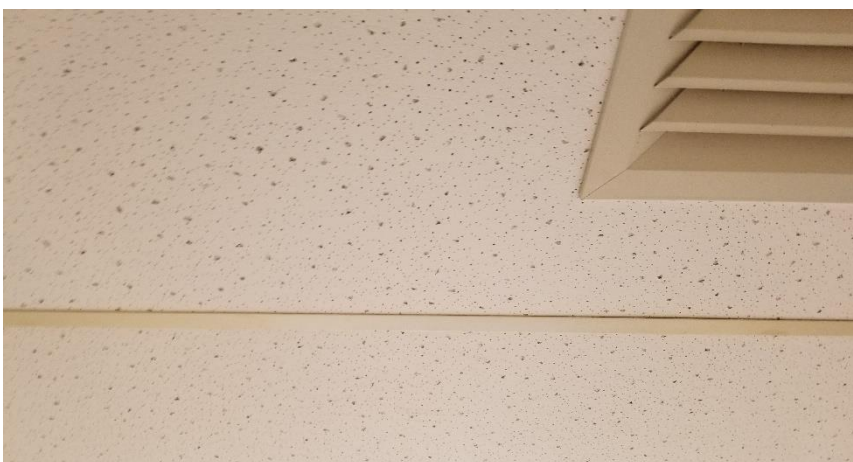
Photo 21: View of the asbestos containing ceiling tiles - 2'x4' Pinholes w/ Triangular Fissures observed in good condition in Room 327.
