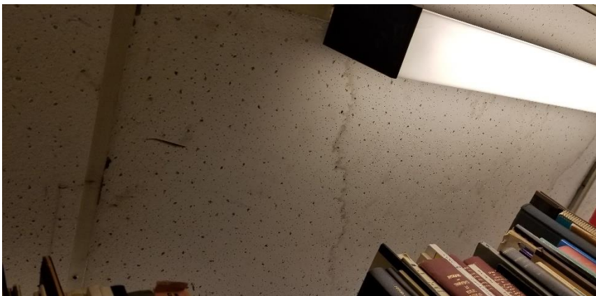
Photo 9: View of the asbestos containing ceiling tiles - 2'x4' Pinholes w/ Triangular Fissures observed in fair condition in Room 523.
