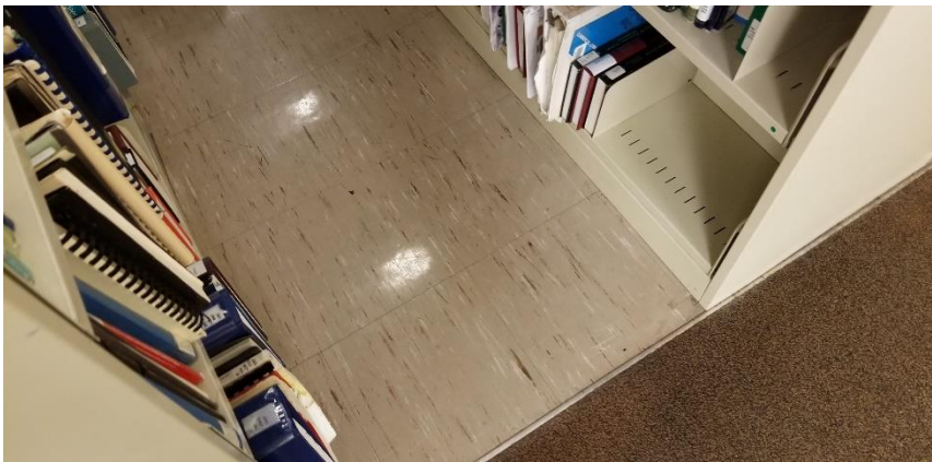
Photo 8: View of the asbestos-containing vinyl floor tiles (12"x12" – Brown w/ Brown Stripes) observed in good condition in Room 523.
