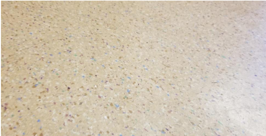
Photo 22: View of the non-asbestos VFT (12"x12" - Pink w/ Multicolour Streaks) observed in Room 223.
