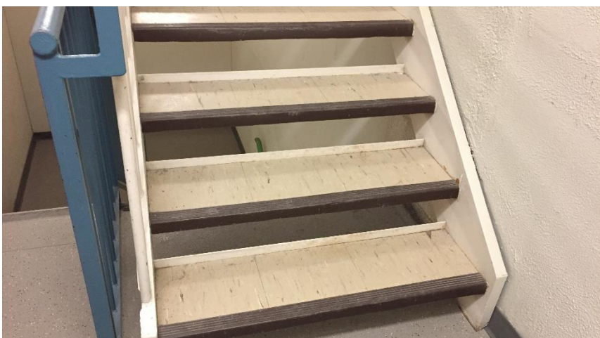
Photo 3: View of the asbestos-containing vinyl floor tiles (12"x12" Beige w/ Grey Streaks) observed in Room 361.
