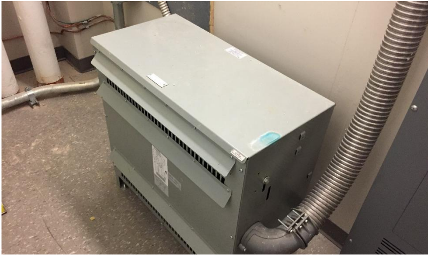
Photo 10: Representative view of the non-PCB dry-type transformers observed throughout the subject building.
