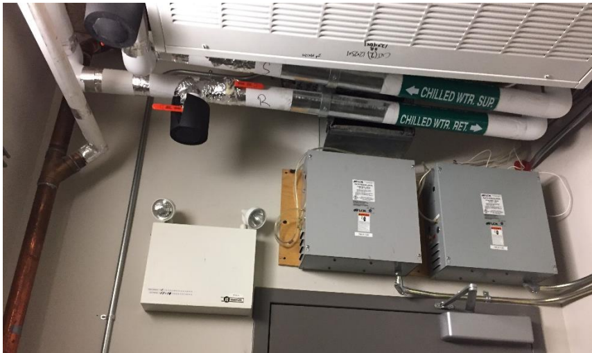
Photo 7: View of the lead-containing battery packs observed in Room 154.
