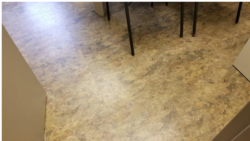
Photo 8: View of the non-asbestos vinyl sheet flooring observed throughout the subject building.
