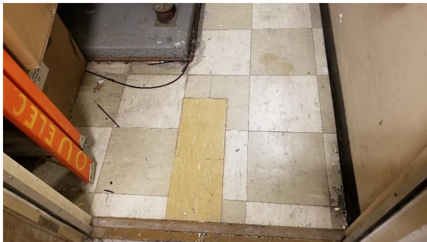
Photo 9: View of the asbestos-containing vinyl floor tiles: (12"x12" – Gold w/ White Streaking), (12"x12" – Grey w/ Streaks), and (12"x12" – Beige w/ Streaks) observed in Room 107J.
