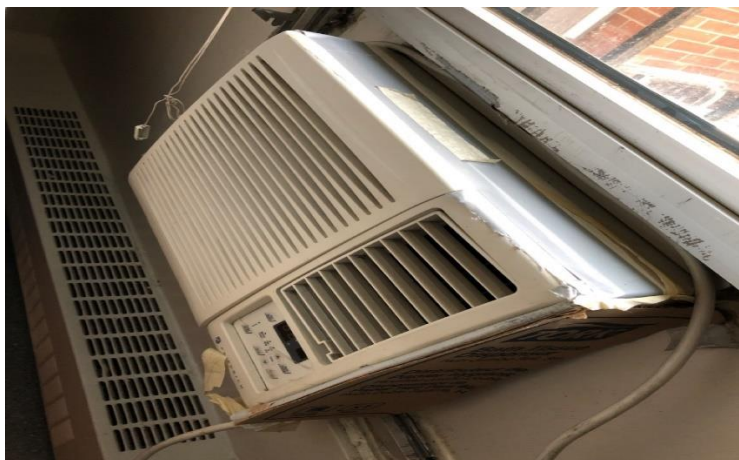
Photo 7: Typical view of ODS containing air-conditioning unit.
