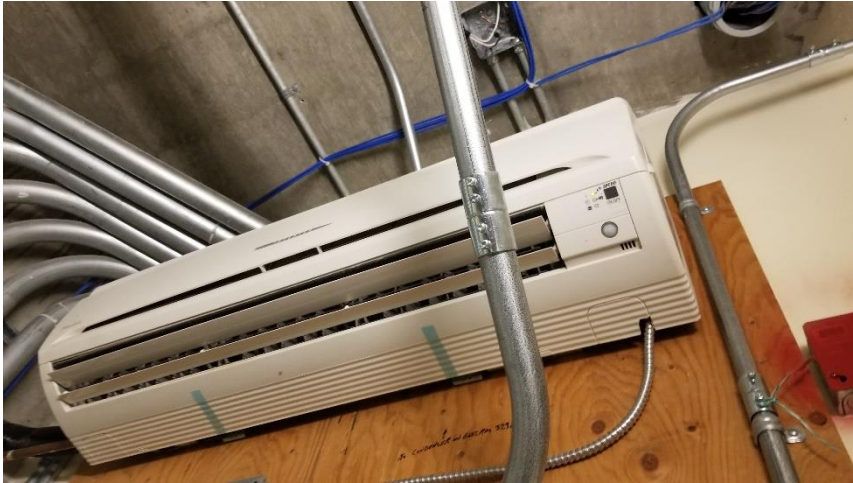
Photo 22: View of the equipment containing ODSs observed in Room 331A.
