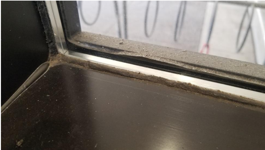
Photo 14: View of the asbestos-containing window glazing (Black) identified in Room 105.
