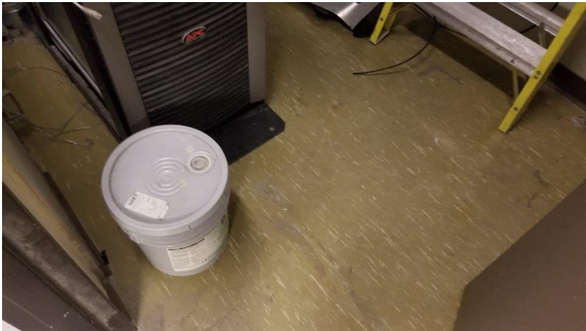
Photo 23: View of the asbestos-containing vinyl floor tiles (12"x12" Green w/ White Striped) observed in good condition in Room 331A.
