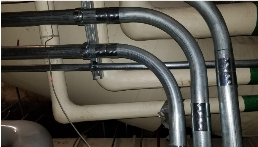
Photo 4: Representative view of the asbestos containing pipe elbow/fitting insulation (parging cement) observed in good condition throughout Room 01 and Room 01B.
