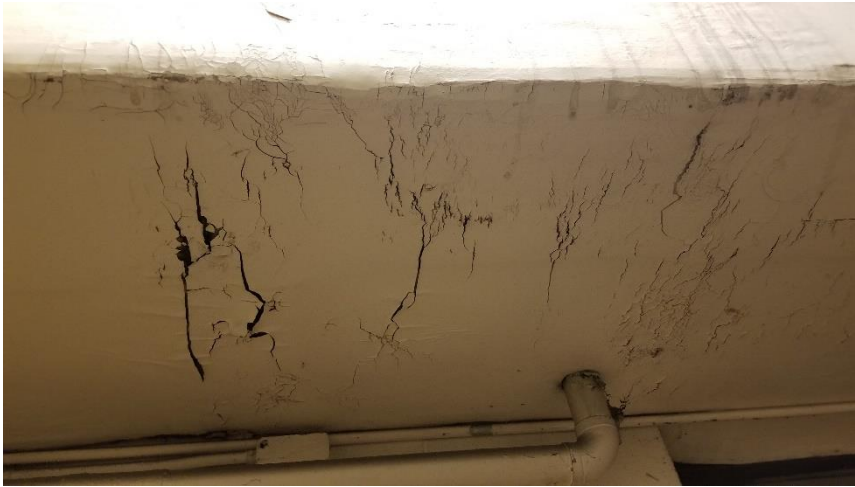
Photo 31: View of the lead-containing paint (Cream) observed in poor condition in Room 500A.
