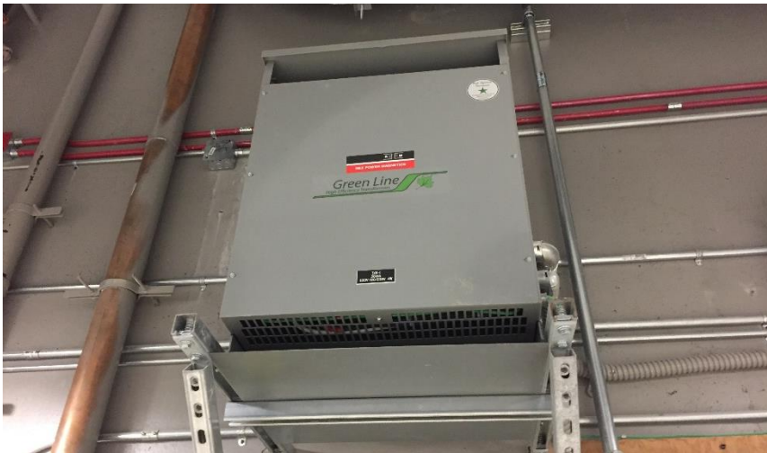
Photo 8: Representative view of the dry-type transformers observed in C043.
