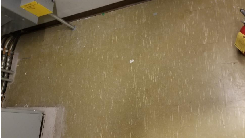
Photo 25: View of the asbestos-containing vinyl floor tiles (12"x12" Green w/ White Striped) observed in good condition in Room 329A.
