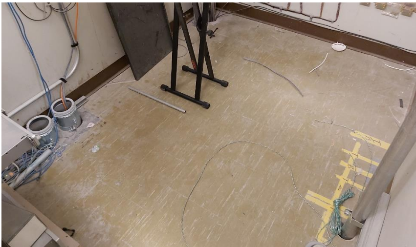
Photo 20: View of the asbestos-containing vinyl floor tiles (12"x12" Green w/ White Striped) observed in good condition in Room 262A.
