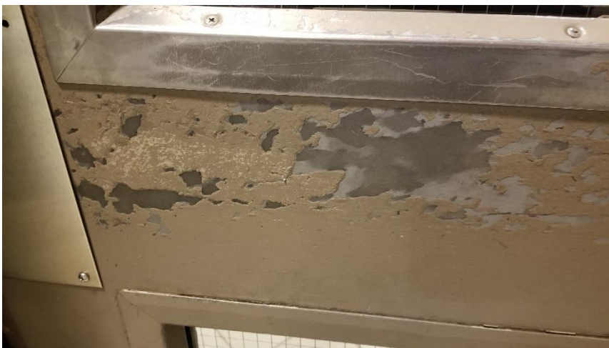
Photo 9: View of the lead-containing door point (Beige) observed in fair condition throughout the first floor.
