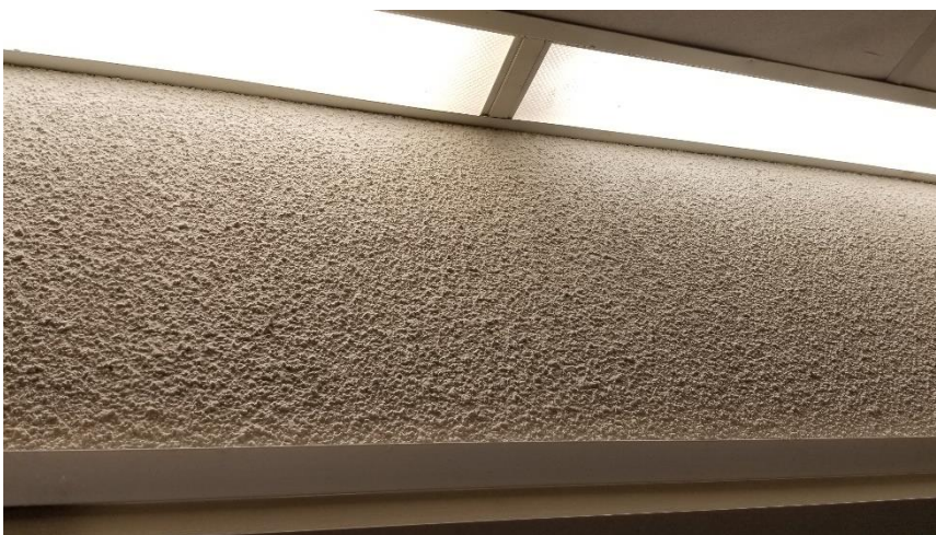
Photo 30: View of the non-asbestos containing wall texture coat observed throughout the 4 th floor.
