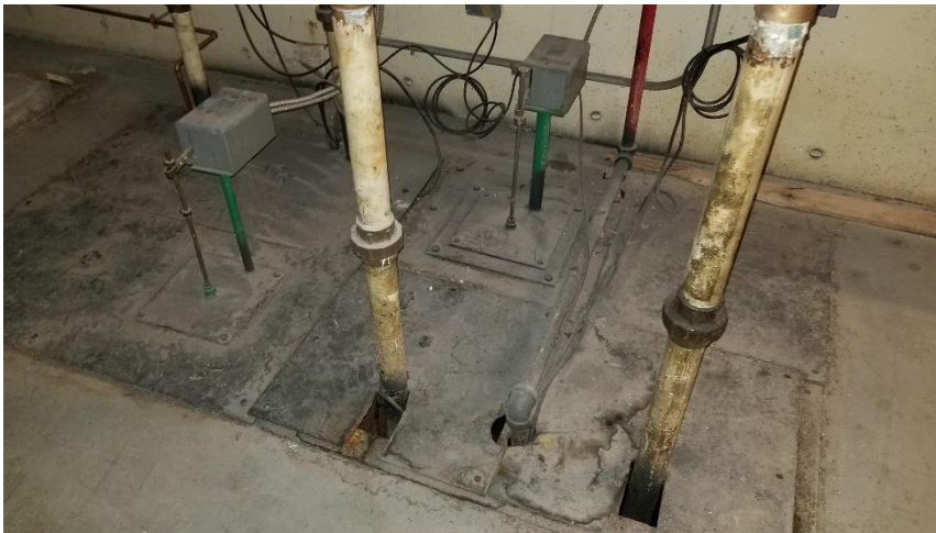
Photo 2: Representative view of the float switches suspected of containing mercury, observed in Room 01.
