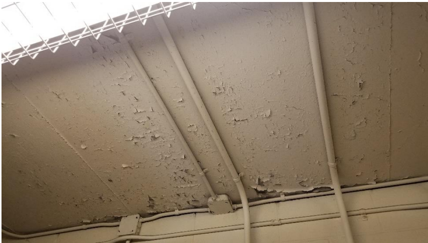
Photo 32: View of the lead-containing paint (Cream) observed in poor condition throughout Room 500B.
