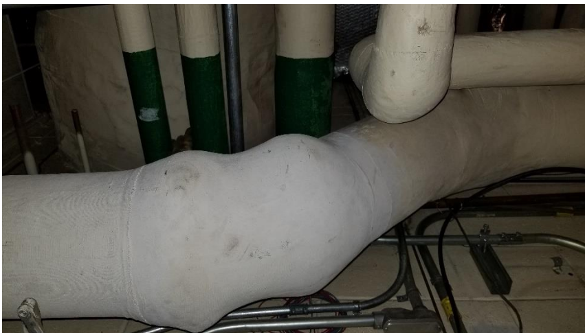
Photo 3: Representative view of the asbestos containing pipe elbow/fitting insulation (parging cement) observed in good condition throughout Room 01 and Room 01B.
