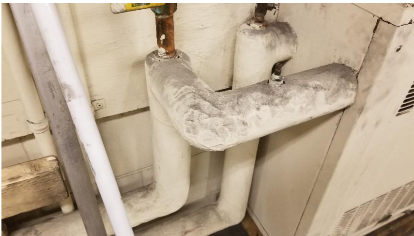
Photo 33: View of the asbestos-containing pipe elbow/fitting insulation (parging cement) observed in good condition in Room 500B.
