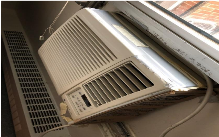
Photo 12: Typical view of ODS containing air-conditioning unit.
