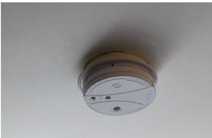
Photo 11: Typical view of smoke detectors containing radioactive materials.
