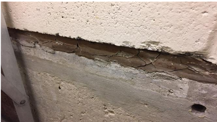
Photo 5: View of asbestos-containing wall caulking (tan) observed in Room 0024.
