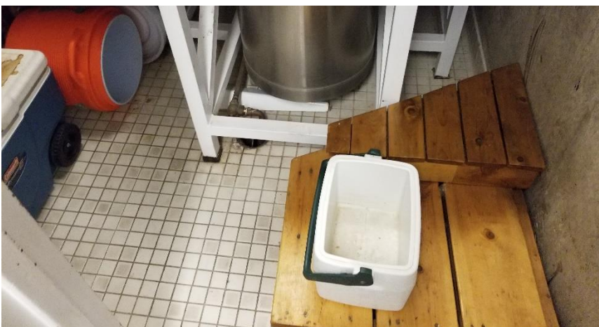
Photo 11: View of ceramic floor tiles grout observed throughout the subject building suspect to contain asbestos.
