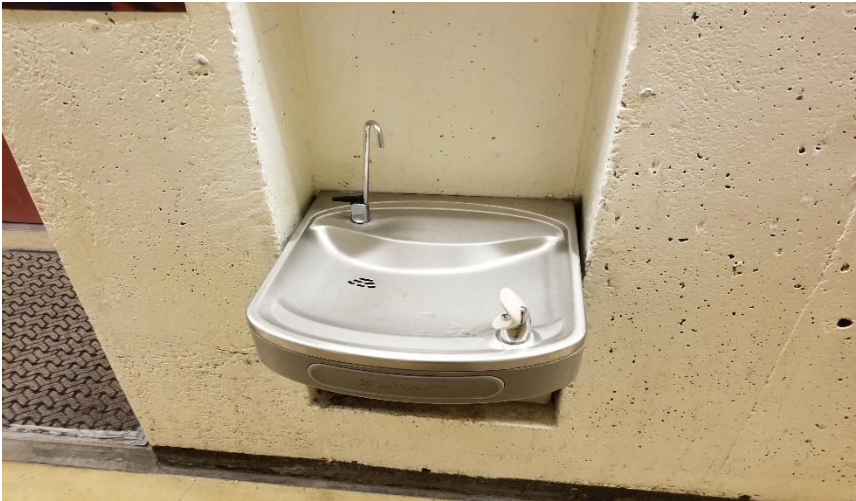
Photo 12: Typical view ODS containing water fountains observed throughout the subject building.
