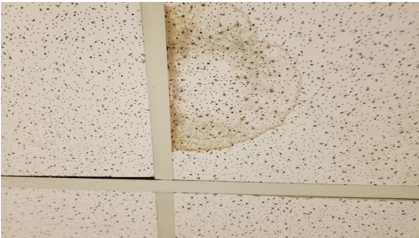
Photo 13: View of water damaged suspended ceiling tile observed in Room 039B.
