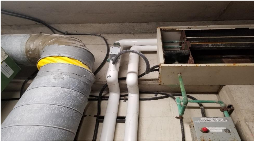
Photo 6: View of flexible duct connector observed in Room 020C suspected to contain asbestos.
