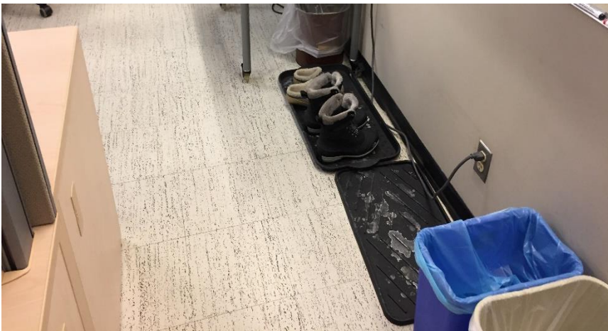
Photo 2: View of asbestos-containing vinyl floor tiles observed in Room 428.
