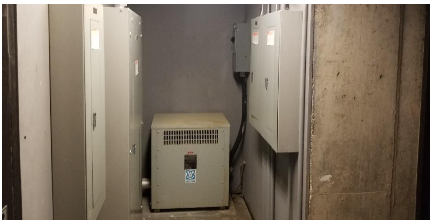
Photo 24: View of the dry-type Westinghouse transformers observed in Room 510.
