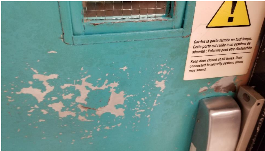
Photo 16: View of the lead containing blue door paint observed in poor condition in Room 217.
