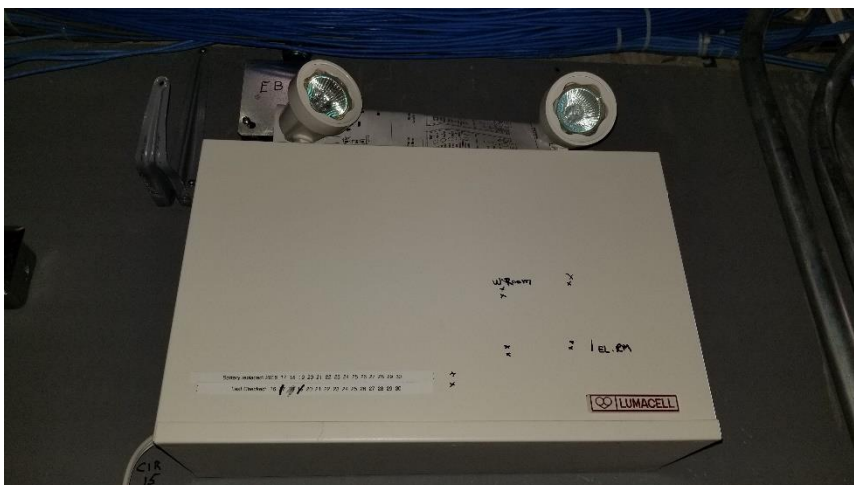
Photo 21: Representative view of the emergency lights containing lead batteries observed in Room 306.
