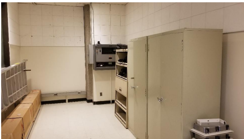
Photo 18: View of the asbestos-containing glue-on acoustic walls tiles observed in good condition in Room 255.
