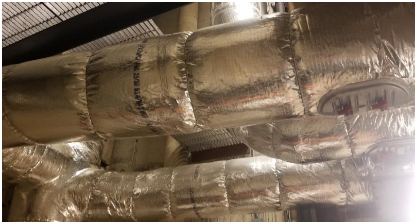
Photo 22: Representative view of the fiberglass insulation observed in Room 431 and 431A.
