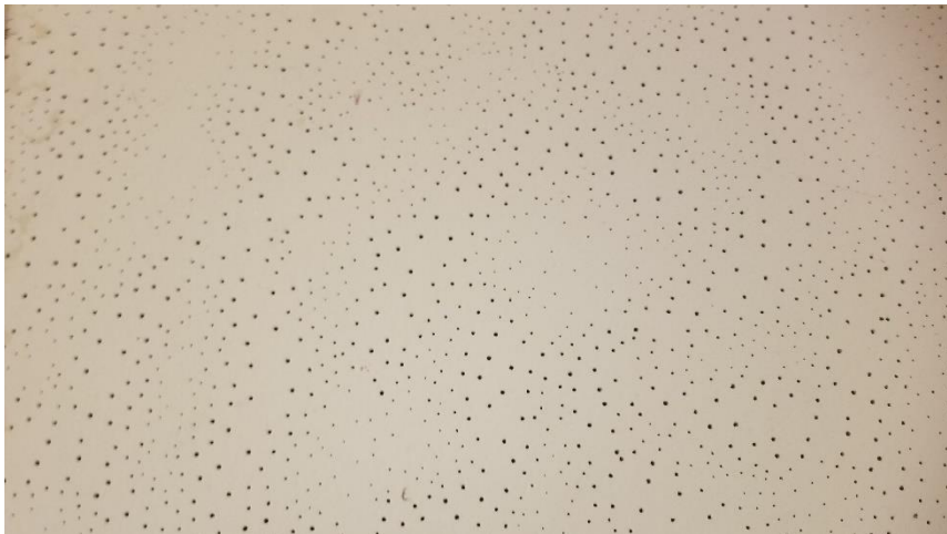
Photo 28: View of the asbestos-containing ceiling tiles (Beige w/ Varying Pinholes) observed and sampled in Room 600G.
