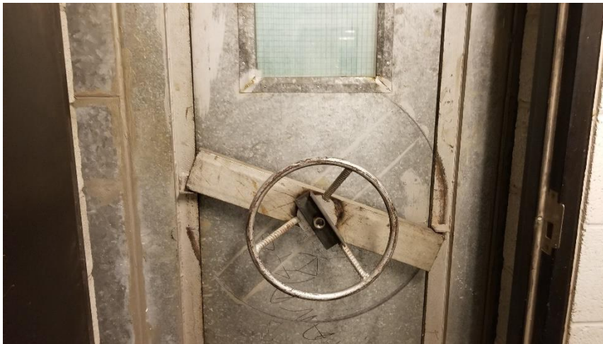
Photo 4: Representative view of the AHU unit doors, with non-asbestos containing thermal insulation in Room 0042.
