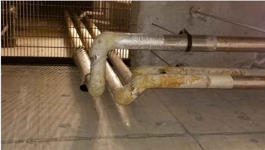
Photo 10: View of the asbestos-containing parging cement elbows/fitting observed in good condition in Room 0032.
