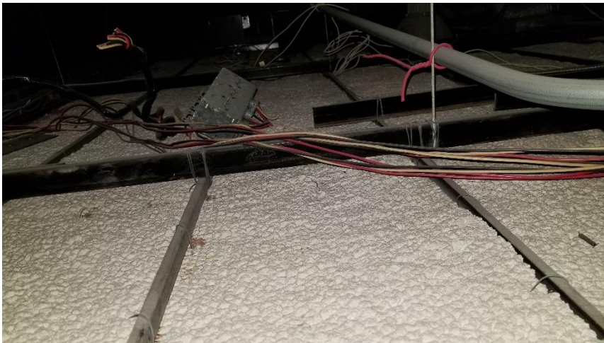
Photo 14: View of the ceiling space above the asbestos-containing ceiling plaster observed in Room 218.
