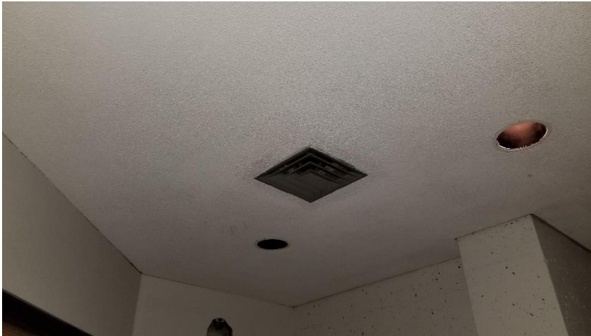
Photo 13: View of the asbestos-containing textured ceiling observed in good condition in Room 218A.
