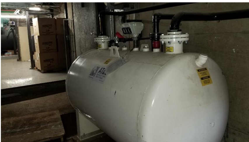
Photo 12: View of the above ground diesel tank observed in Room 0042D.
