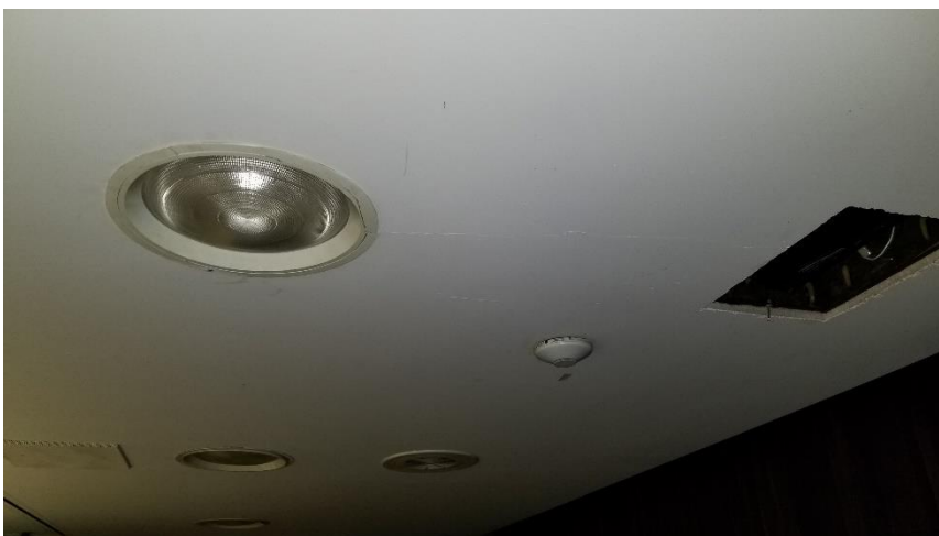
Photo 15: View of the asbestos-containing ceiling plaster observed in Room 218D, with poor condition areas.
