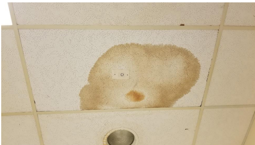
Photo 9: View of the water damaged asbestos-containing ceiling tile observed in Room 0021.
