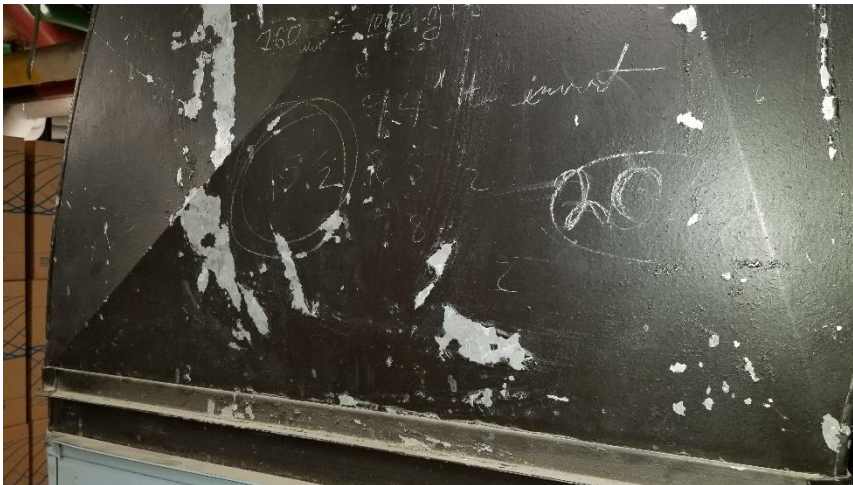
Photo 11: Representative view of the lead containing Black mechanical equipment paint observed throughout Room 0042 in poor condition.
