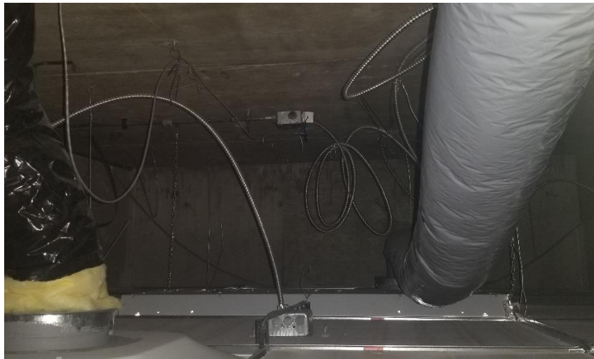
Photo 29: Representative view of the bare concrete ceiling finishes observed above suspended ceiling tiles in Room 602.
