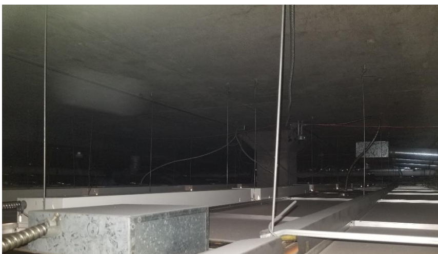
Photo 27: Representative view of the bare concrete ceiling finishes observed above suspended ceiling tiles in Room 600G.
