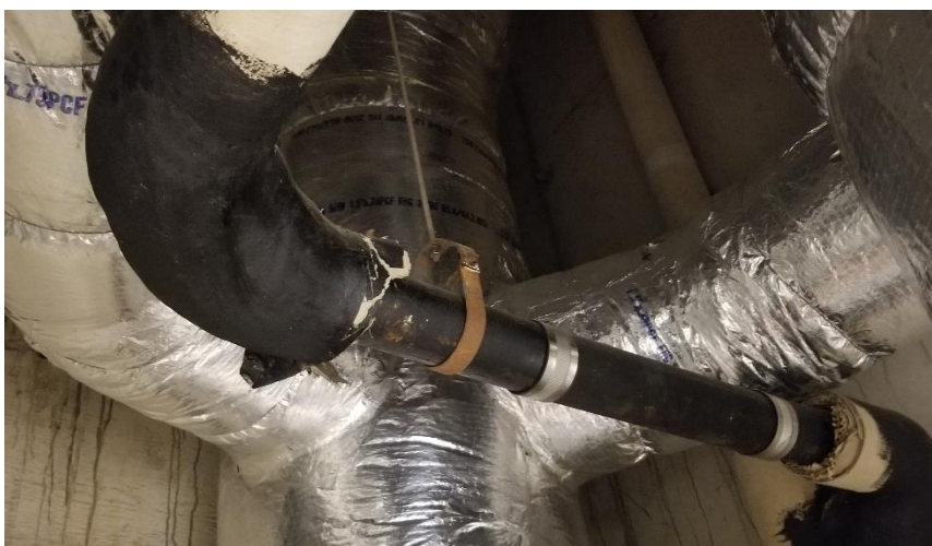
Photo 30: View of the poor condition asbestos-containing pipe straight insulation observed in Room 622A.
