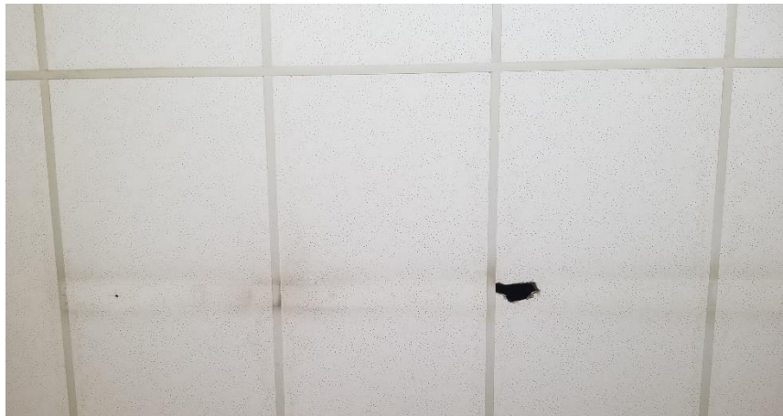
Photo 31: View of the asbestos-containing ceiling tiles (Beige w/ Varying Pinholes) observed with damages in Room 621.
