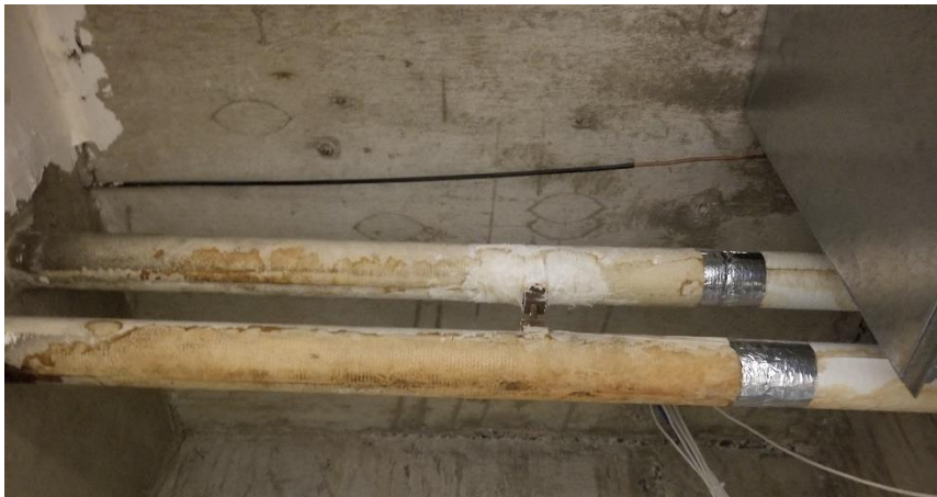
Photo 25: View of the water damaged fiberglass pipe straight insulation observed in Room 510A.
