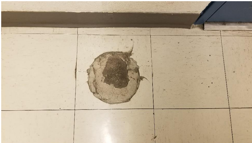
Photo 7: Previously identified vinyl floor tiles (12"x12" – White w/ Brown Flakes) observed in poor condition in Room 001.
