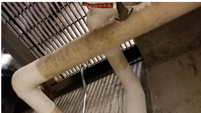
Photo 23: View of the asbestos-containing piping cement elbows observed in good condition in Room 506A.
