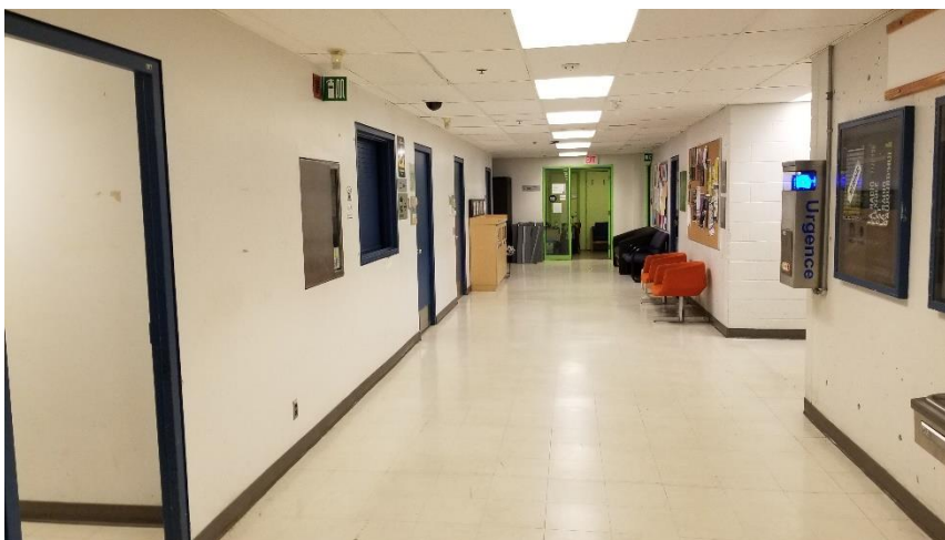
Photo 6: Representative view of Room 001, containing asbestos vinyl floor tiles (12"x12" - White w/ Brown Flakes).
