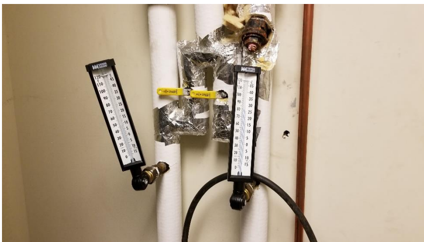
Photo 3: Representative view of the pressure gauges containing liquid mercury observed in Room 038E.
