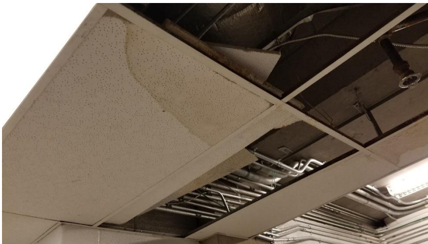
Photo 8: View of the suspended ceiling tiles (2'x4' – Pinholes w/ Large Fissures) observed to be manufactured in 1996 in Room 001A. Water staining was observed on select tiles.
