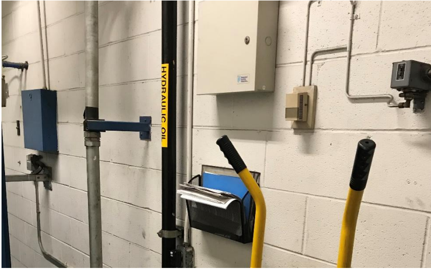
Photo 4: View of mercury-containing thermostat switches observed throughout the subject building.
