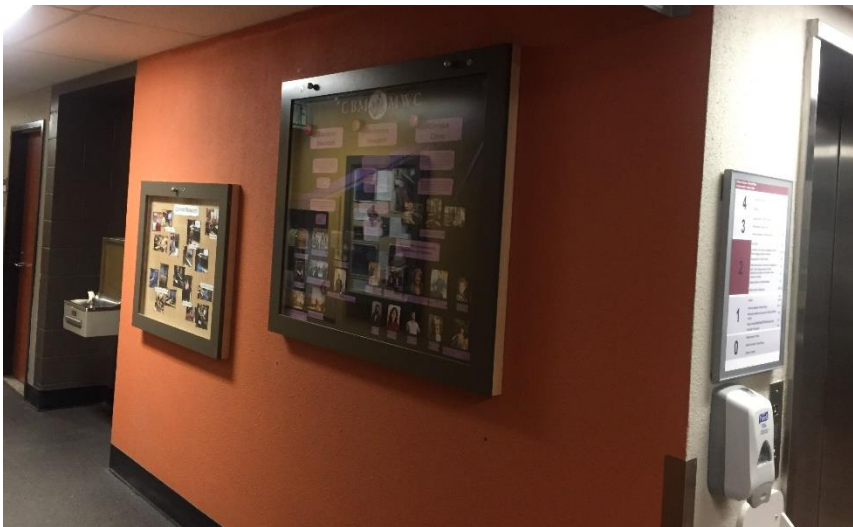
Photo 2: Representative view of the wall texture coat (painted orange) in Room 200, containing 10% Chrysotile asbestos.
