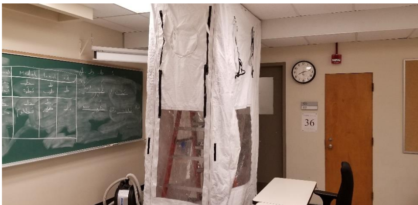
Photo 30: Representative view of the Type 2 ceiling entries performed during the site survey to access ceiling spaces.
