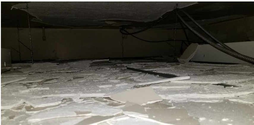
Photo 17: Representative view of the asbestos-containing ceiling plaster debris observed on suspended ceiling tiles throughout Room 206.
