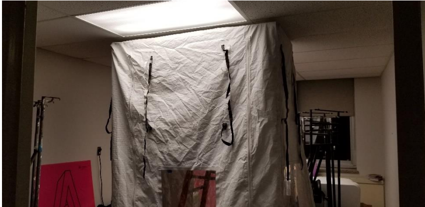
Photo 28: Representative view of the Type 2 ceiling entries performed during the site survey to access ceiling spaces.
