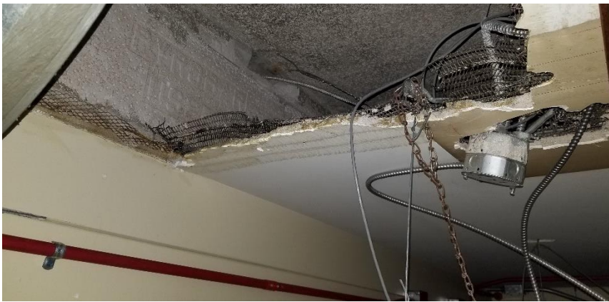
Photo 26: View of the poor condition asbestos-containing ceiling plaster and overspray observed above the suspended ceiling tiles in Room 403.
