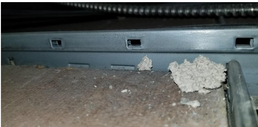
Photo 12: Representative view of the asbestos-containing ceiling plaster debris observed on suspended ceiling tiles throughout Room 02D.
