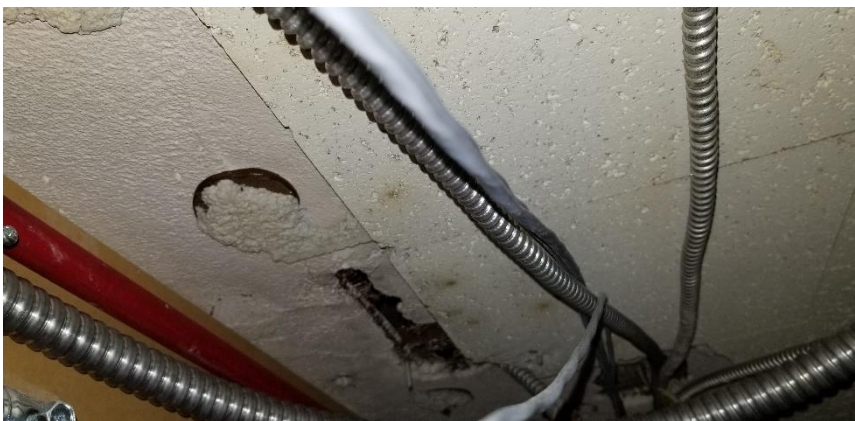
Photo 15: View of the non-asbestos acoustic glue-on tiles and mastic pucks (Dark Brown) observed overtop the ceiling plaster throughout Level 0.
