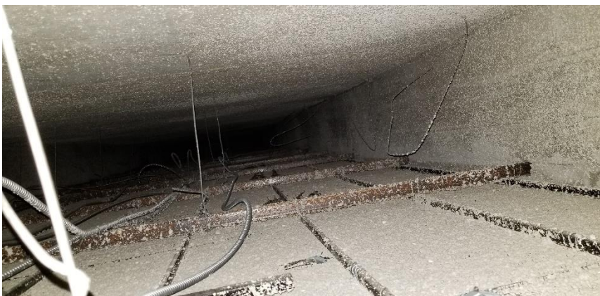
Photo 21: View of the asbestos-containing ceiling plaster and overspray observed above the suspended ceiling tiles in Room 303.
