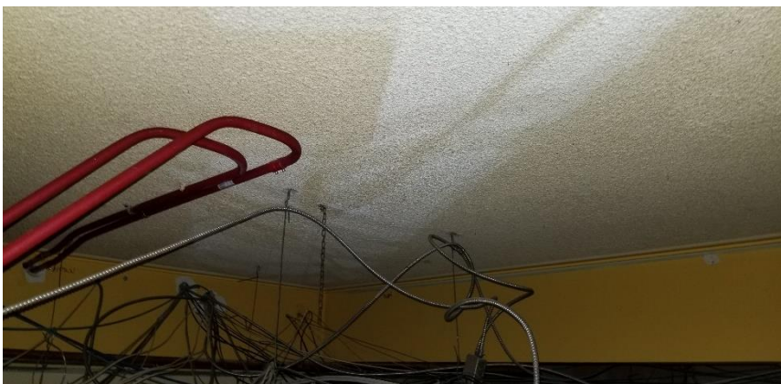
Photo 9: View of the asbestos-containing ceiling plaster observed above the suspended ceiling tiles in Room 02.
