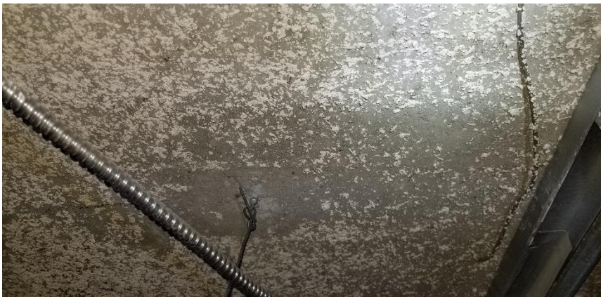
Photo 11: Representative view of the asbestos-containing sprayed-on ceiling plaster overspray observed on adjacent building materials and equipment observed throughout Room 02D.
