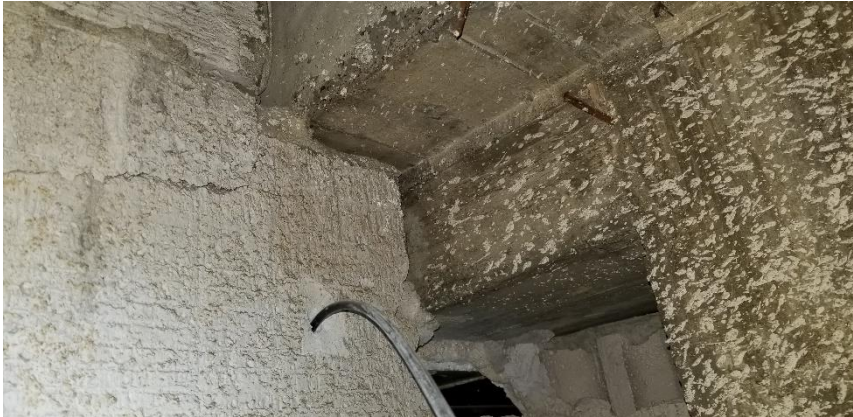
Photo 25: View of the asbestos-containing plaster overspray observed on walls along the Room 401B hallway.
