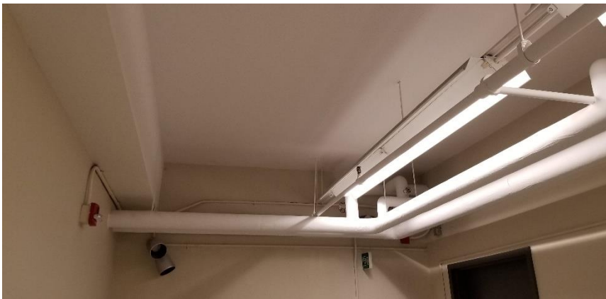
Photo 8: Representative view of the asbestos-containing parging cement elbows observed in good condition throughout Room 002.
