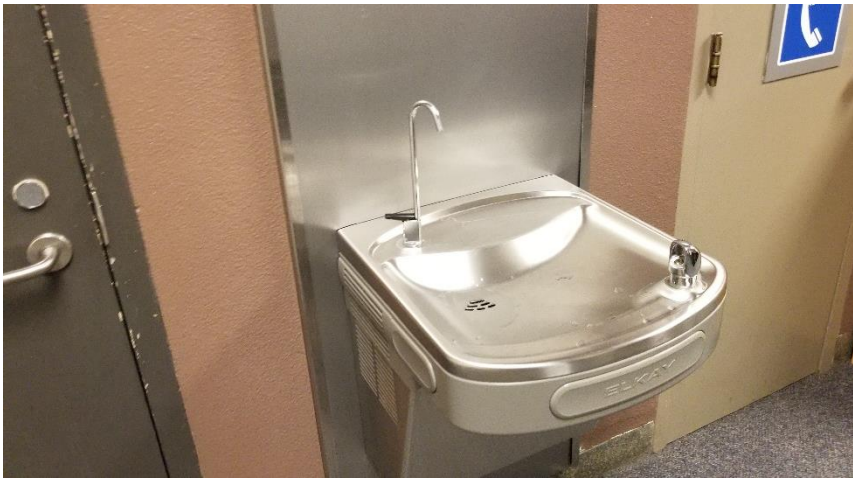
Photo 20: Representative view of water fountains observed throughout the subject building, containing ODSs (R134a).
