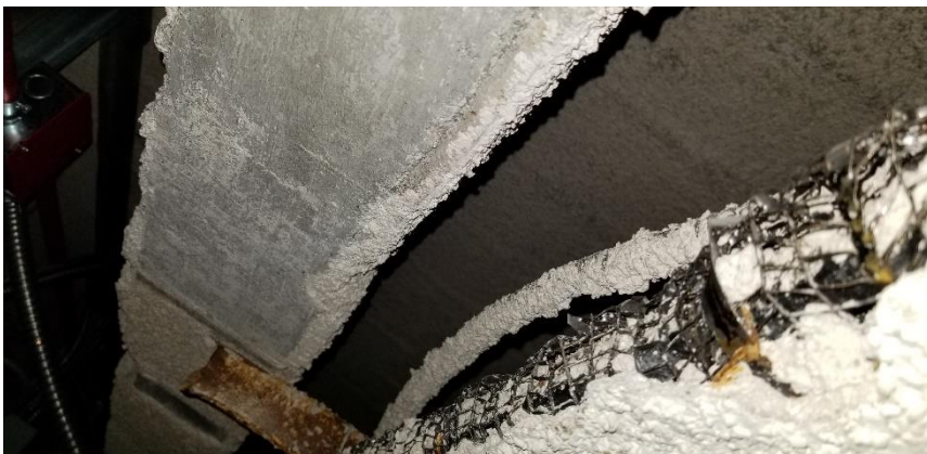
Photo 24: View of the poor condition asbestos-containing ceiling plaster and overspray observed above the suspended ceiling tiles in Room 423.
