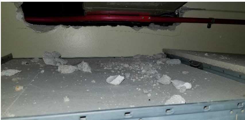
Photo 27: Representative view of the asbestos-containing ceiling plaster debris observed on suspended ceiling tiles throughout Room 403.
