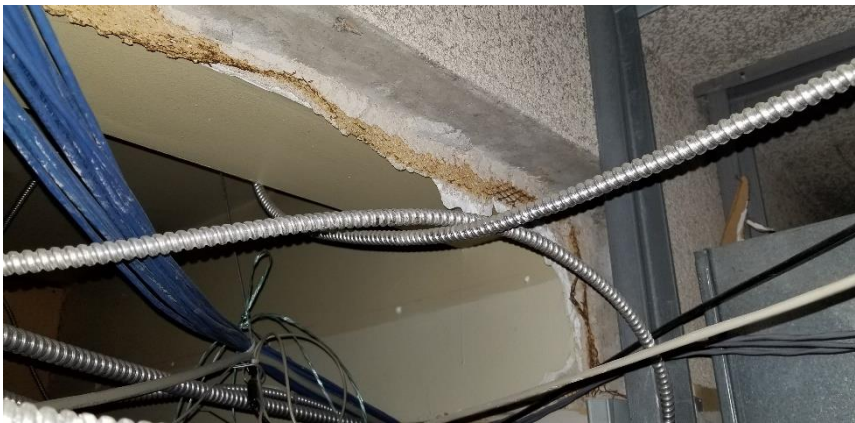
Photo 14: Representative view of the damaged asbestos-containing plaster observed throughout the subject building.
