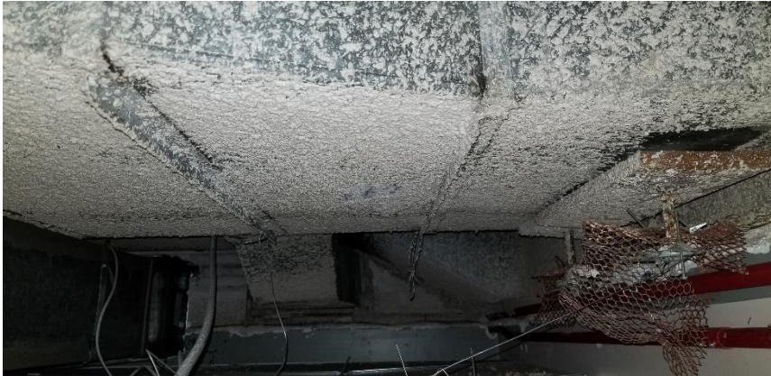
Photo 16: Representative view of the asbestos-containing sprayed-on ceiling plaster overspray observed on adjacent building materials and equipment observed throughout Room 102B.
