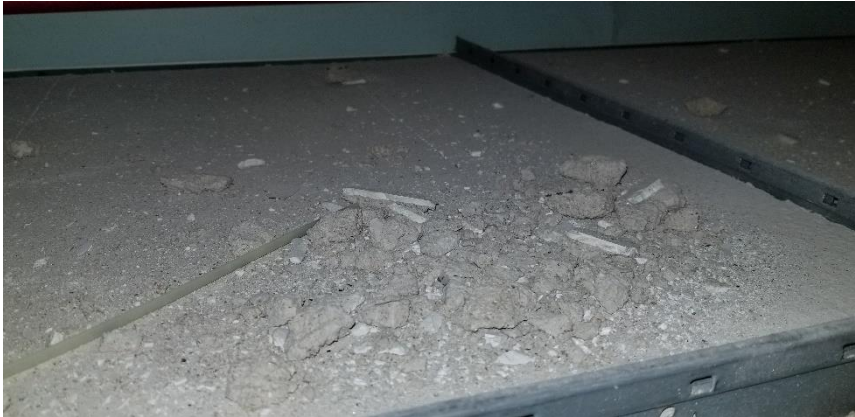
Photo 22: Representative view of the asbestos-containing ceiling plaster debris observed on suspended ceiling tiles throughout Room 303.
