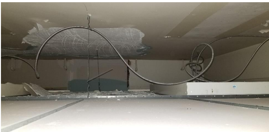
Photo 18: Representative view of the asbestos-containing ceiling plaster debris observed on suspended ceiling tiles throughout Room 212.
