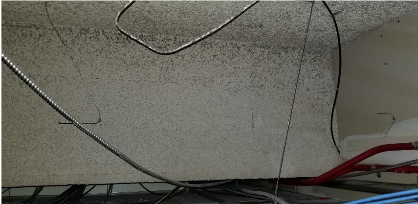
Photo 10: Representative view of the asbestos-containing sprayed-on ceiling plaster overspray observed on adjacent building materials and equipment observed throughout Room 02D.
