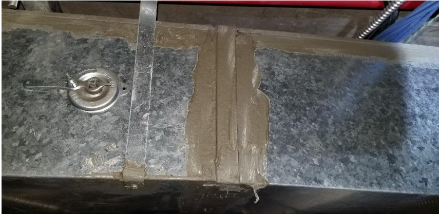
Photo 13: View of the non-asbestos-containing HVAC duct caulking observed throughout the subject building.
