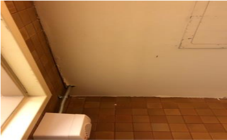
Photo 7: View of asbestos-containing drywall joint compound observed to be in poor condition in Room 047.
