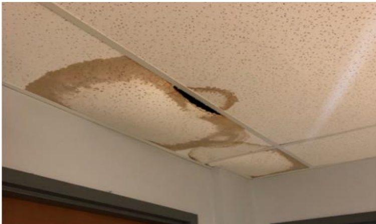
Photo 16: View of water damaged ceiling tiles observed in Room 104.
