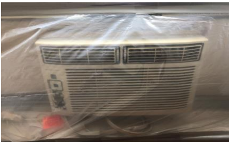
Photo 18: View of ODS containing air-conditioning unit in Room 126E.
