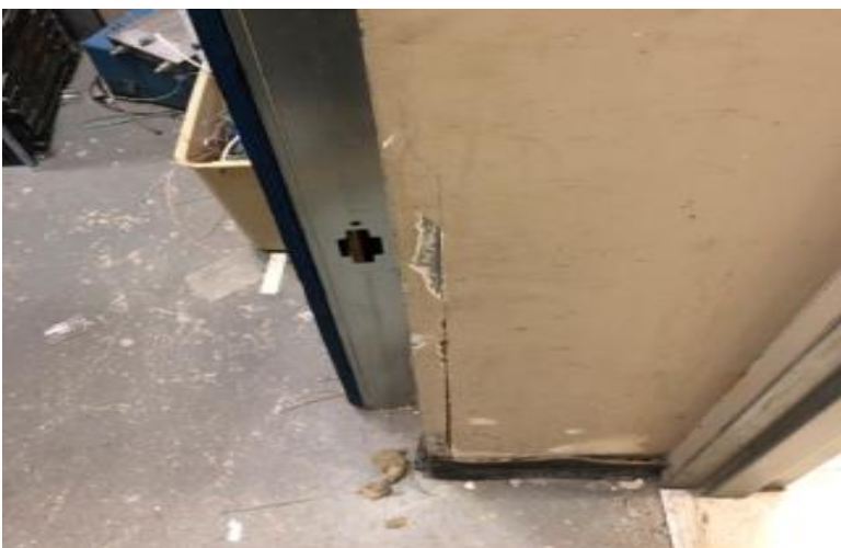
Photo 6: View of asbestos-containing drywall joint compound observed to be in poor condition in Room 03.
