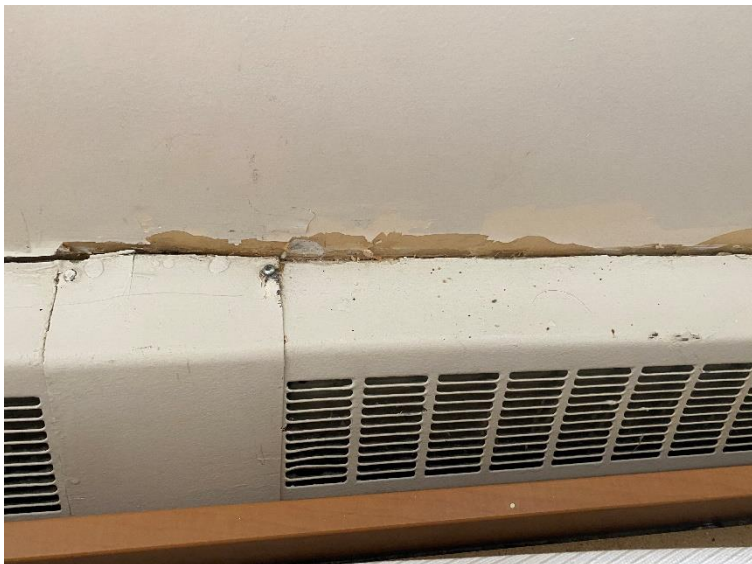
Photo 11: View of asbestos-containing drywall joint compound observed to be in poor condition in Room 315.
