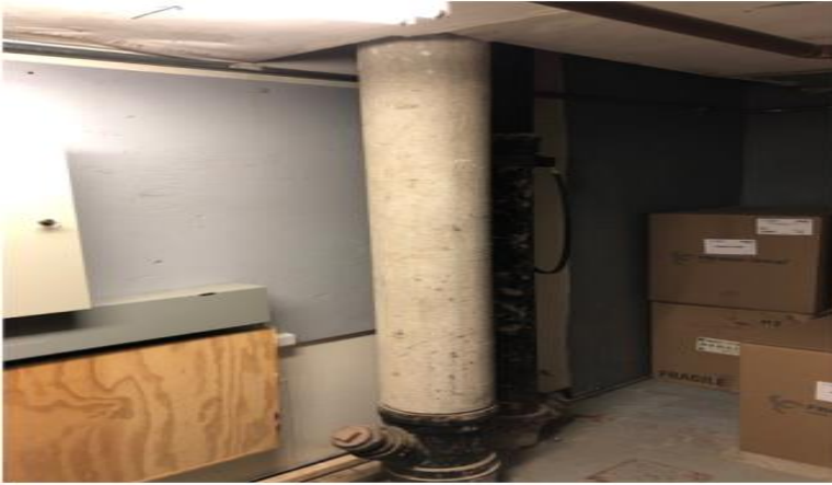
Photo 13: View of asbestos-containing transite pipe observed in Room 045.
