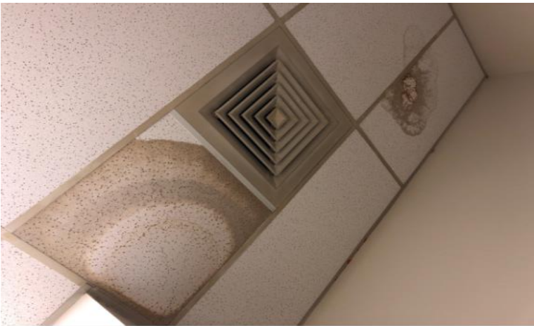
Photo 14: View of water damaged ceiling tiles observed in Room 09.
