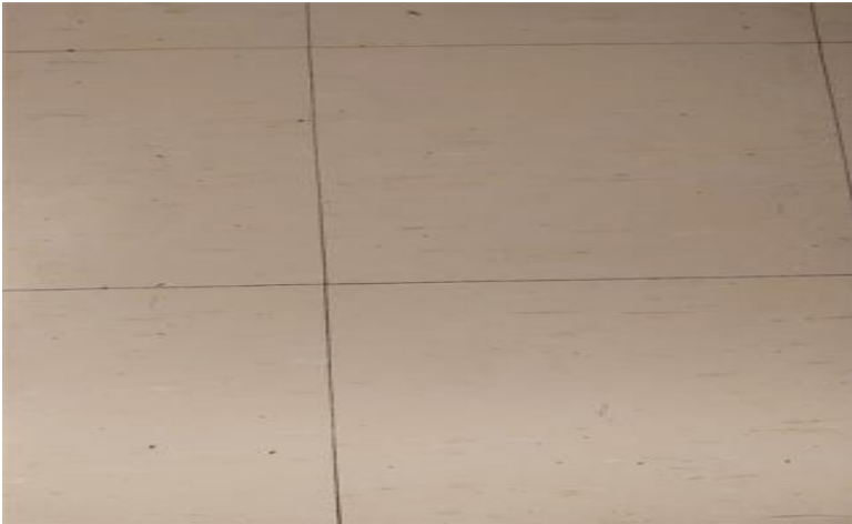
Photo 4: View of asbestos-containing vinyl floor tiles (12"x12" - Beige) observed in Room 1918A.
