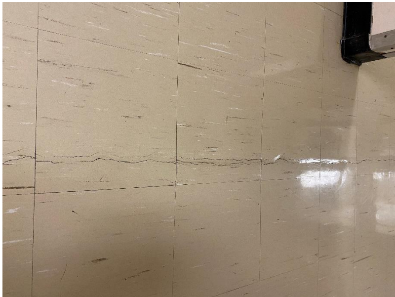
Photo 9: View of asbestos-containing vinyl floor tiles observed to be in fair condition in Room 122.
