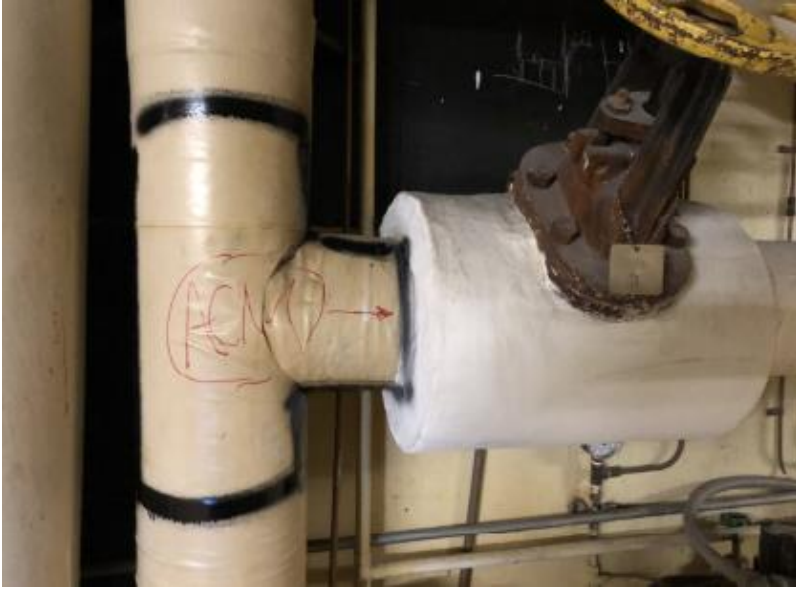
Photo 3: View of asbestos-containing mechanical fitting insulation observed in Tunnel 6-5.
