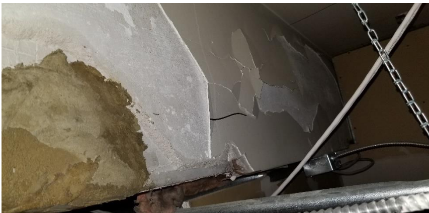
Photo 3: View of asbestos-containing wall plaster observed to be in poor condition in Room 5082.
