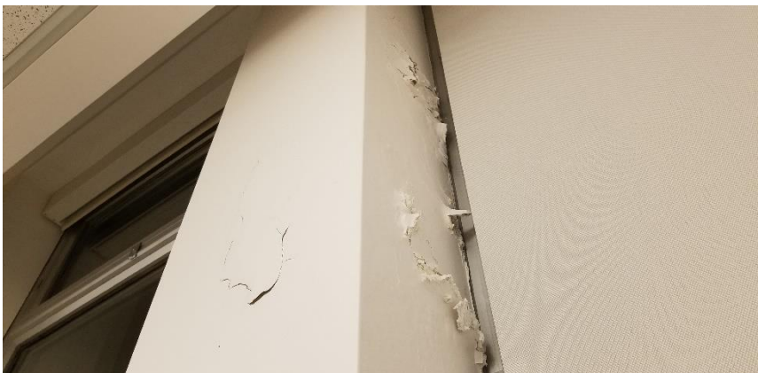
Photo 6: View of asbestos-containing wall plaster observed to be in poor condition Room 1076.
