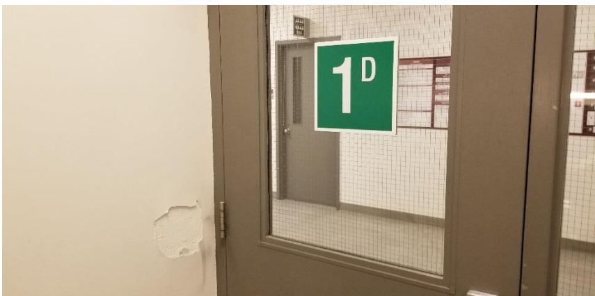
Photo 5: View of asbestos-containing wall plaster observed to be in poor condition in Room 1070.
