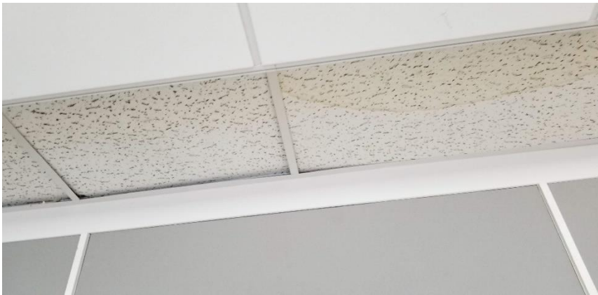
Photo 11: View of water-staining observed on suspended ceiling tiles in Room 5069A.
