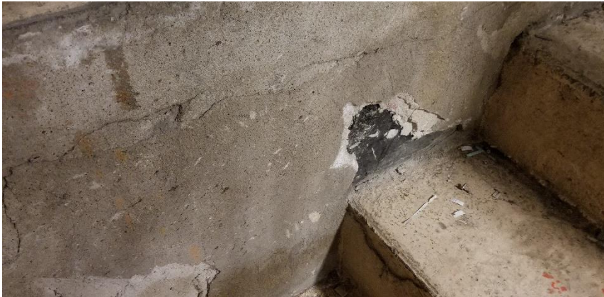
Photo 7: View of asbestos-containing wall plaster observed to be in poor condition in Room 0189.
