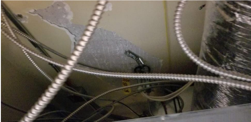
Photo 4: View of asbestos-containing ceiling plaster observed to be in poor condition above the suspended ceiling tiles in Room 1026.
