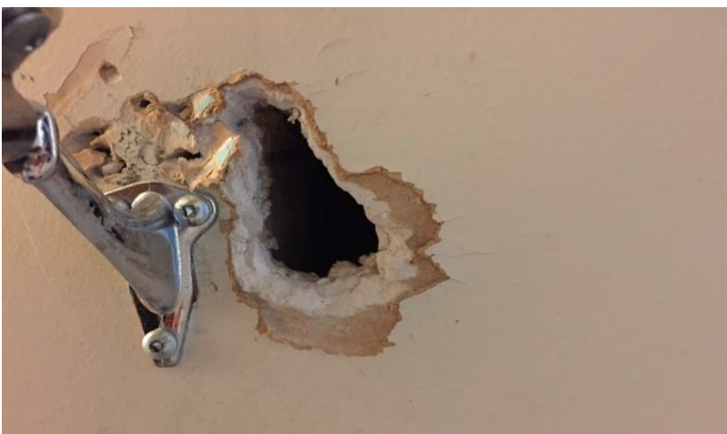
Photo 6: View of damaged asbestos-containing drywall joint compound observed in Room K.
