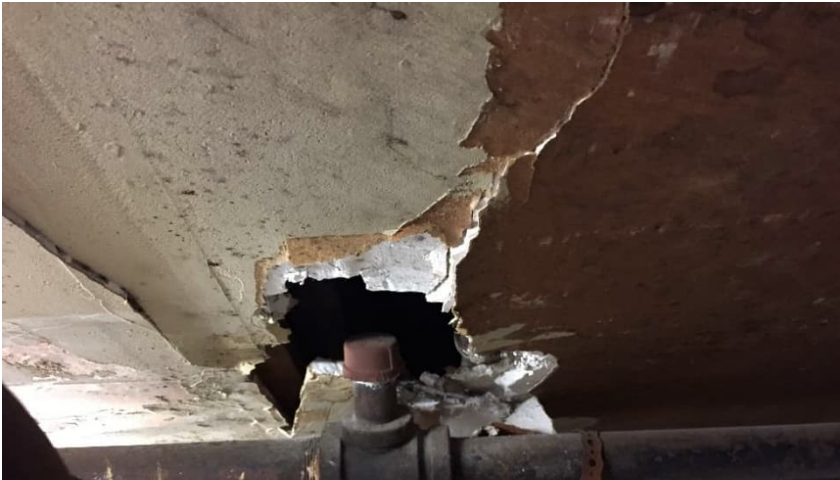
Photo 7: View of damaged asbestos-containing drywall joint compound observed on the basement ceiling.
