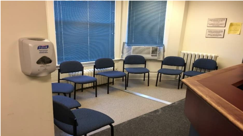
Photo 4: Representative view of asbestos-containing drywall joint compound observed throughout the subject building.
