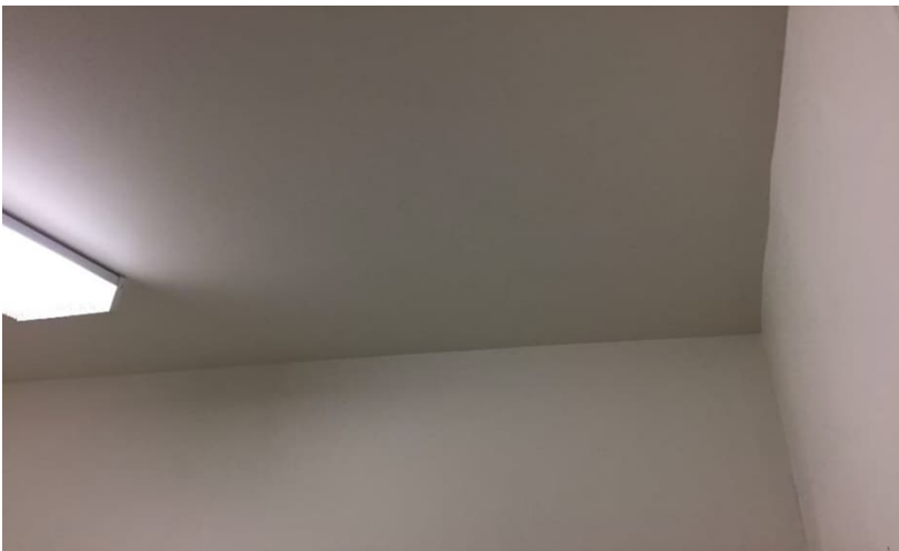
Photo 8: View of lead wall and ceiling paint (White) observed to be in good condition in Room 17.
