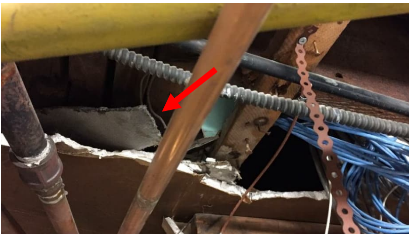
Photo 9: View of the asbestos-containing paper insulation (Grey) observed in poor condition in Room B.
