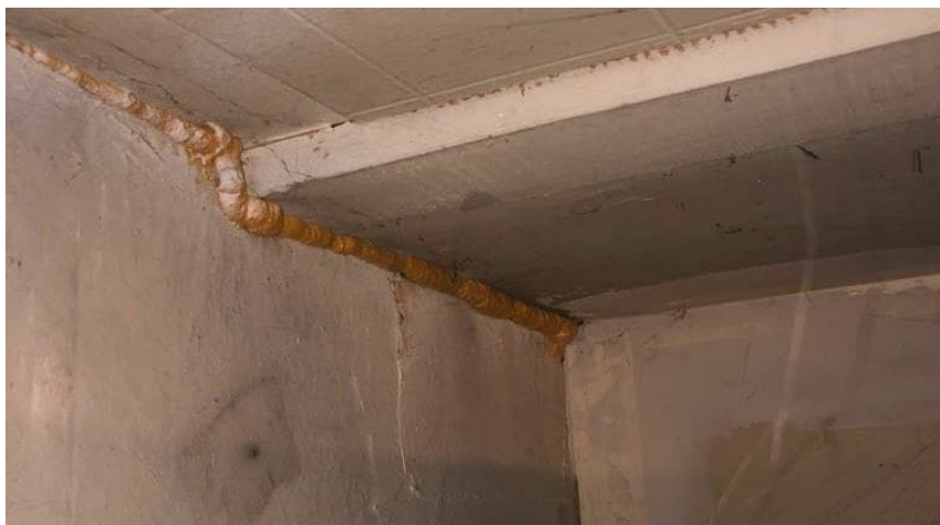
Photo 10: View of the spray foam insulation (Yellow) in which an asbestos-containing fibrous material was identified in Room H.
