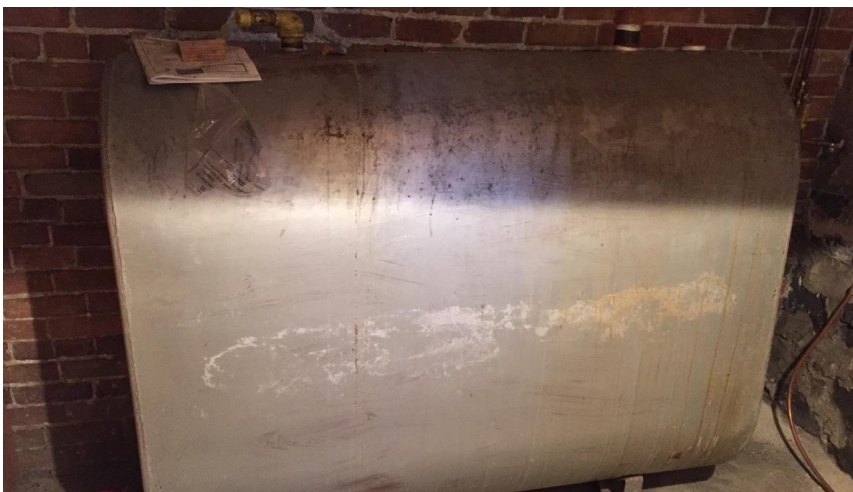
Photo 5: View of the above ground diesel storage tank observed in Room B1.
