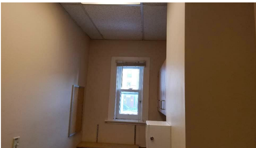
Photo 3: Typical view of finishes on the ground floor including asbestos-containing plaster.
