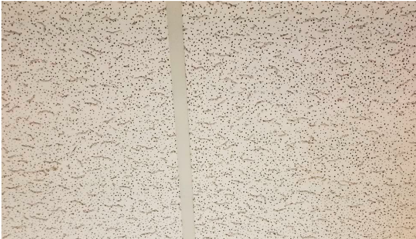
Photo 8: Typical view of non-asbestos suspended ceiling tiles observed throughout the subject building.
