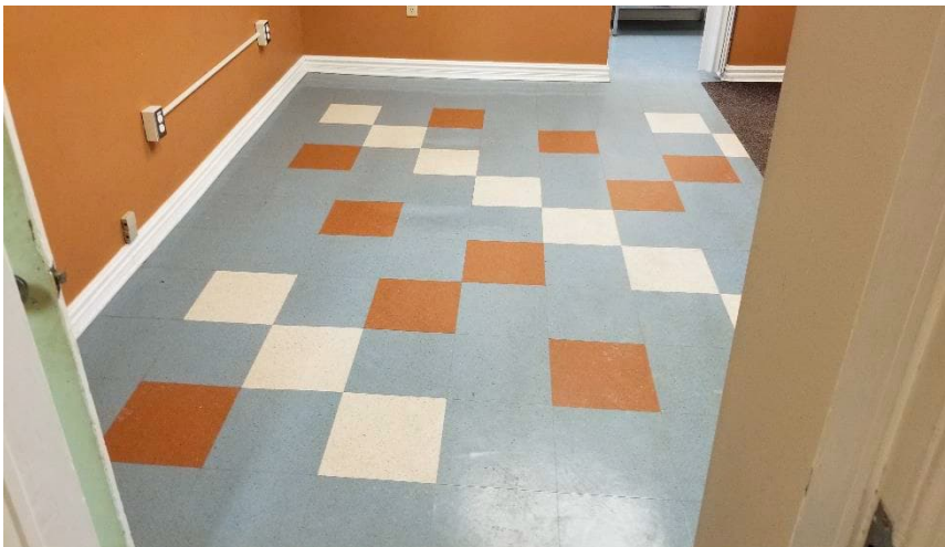
Photo 9: Typical view of non-asbestos vinyl floor tiles (12"x12"- White w/ Red & Blue) observed throughout the subject building.
