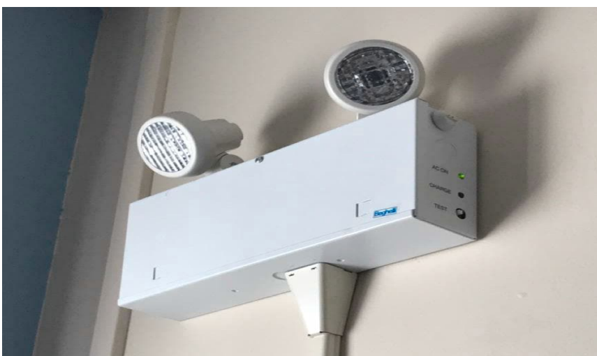
Photo 10: View of lead-containing emergency battery pack observed in Room 206.
