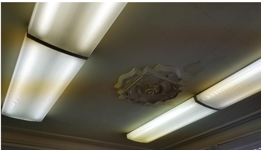
Photo 9: View of lead-containing beige paint observed on the ceiling in Room 102.
