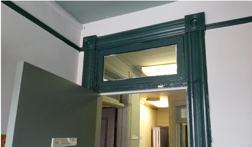
Photo 13: View of lead-containing dark green paint observed on the doorframe of Room 206.
