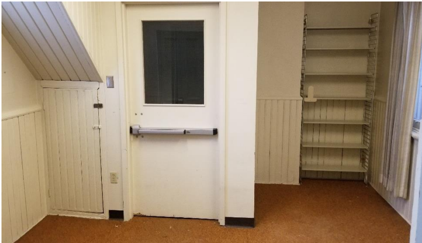
Photo 8: View of lead-containing white paint observed on the wall in Room 105.
