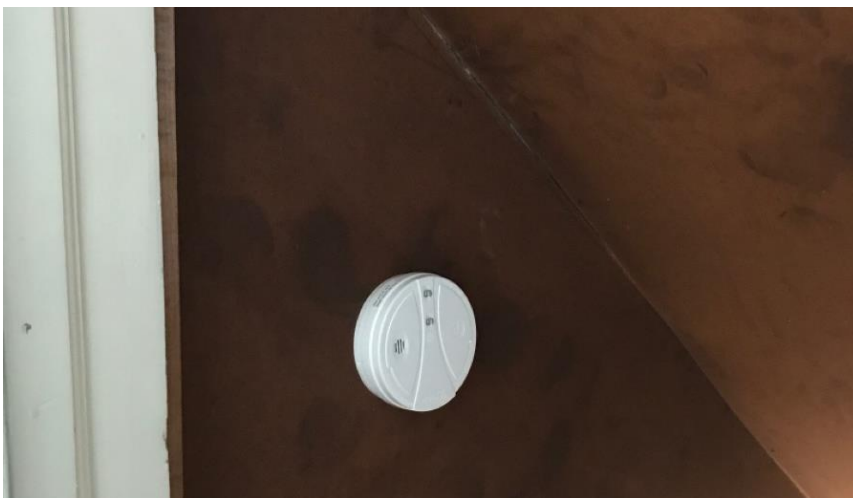
Photo 16: View of radioactive-containing smoke detector observed in Room B3.
