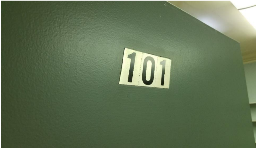
Photo 10: View of lead-containing green paint observed on the door of Room 101.
