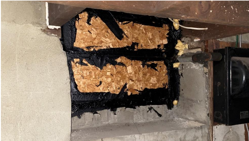
Photo 2: View of asbestos-containing black mastic containing 10% Chrysotile on basement window plywood.
