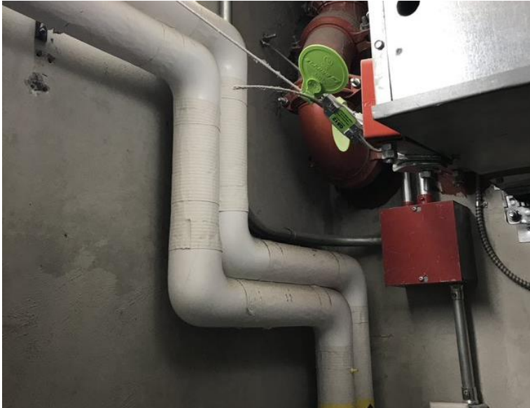
Photo 1: View of fibreglass pipe insulation observed in the parking garage of the subject building.
