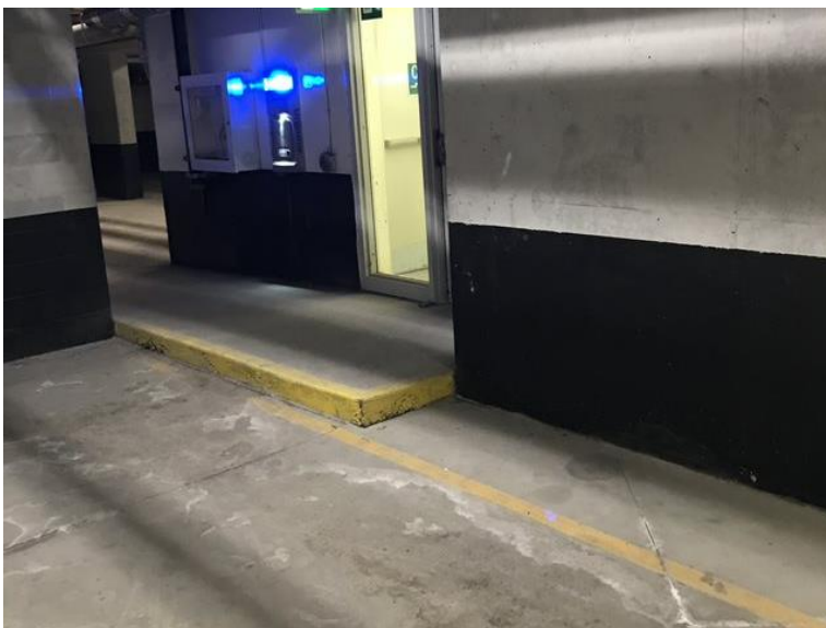
Photo 2: View of the low level lead paints (black and yellow) observed in the parking garage of the subject building.
