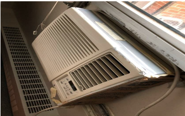
Photo 11: Typical view of ODS containing air-conditioning unit.
