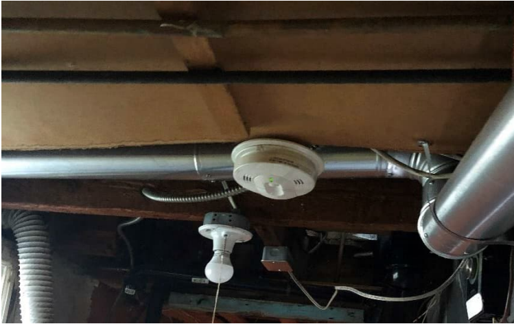
Photo 7: Typical view of smoke detectors containing radioactive material.
