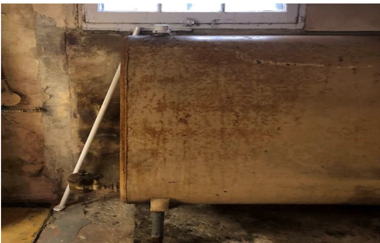
Photo 6: View of AST observed throughout the basement of the subject building (photo taken post-flood remediation work by Xpertek in October 2020).
