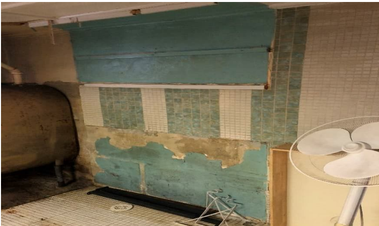
Photo 5: View of lead-containing aqua blue paint observed to be in poor condition on the walls in the laundry room throughout the basement (photo taken post-flood remediation work by Xpertek in October 2020).
