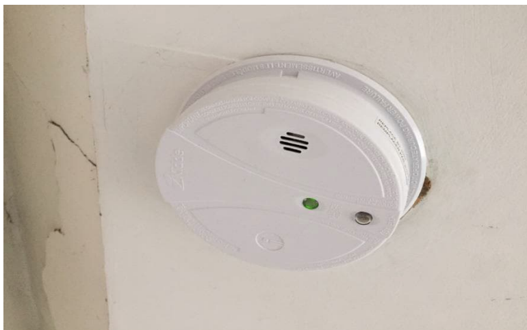
Photo 10: Typical view of smoke detectors containing radioactive materials.
