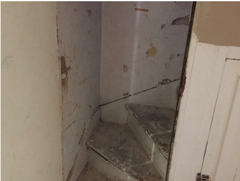
Photo 5: View of asbestos-containing wall plaster observed to be in poor condition in the stairwell to the 3 rd floor of the subject building.
