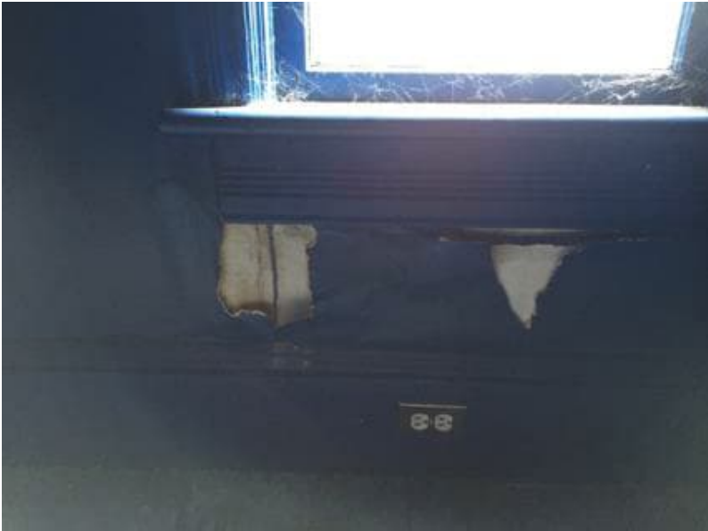
Photo 8: View of lead-containing blue paint observed to be in poor condition on the 3 rd floor of the subject building.
