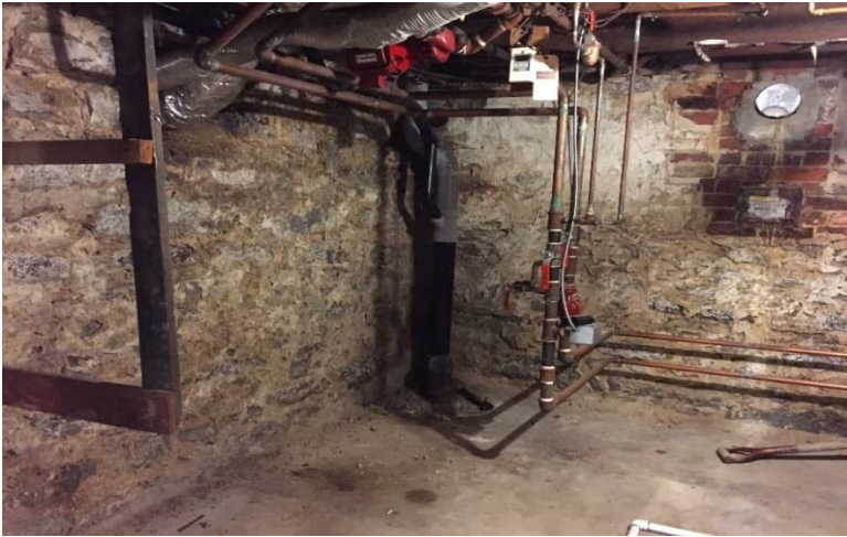
Photo 4: View of typical finishes observed at the building located at 102 Henderson Avenue.
