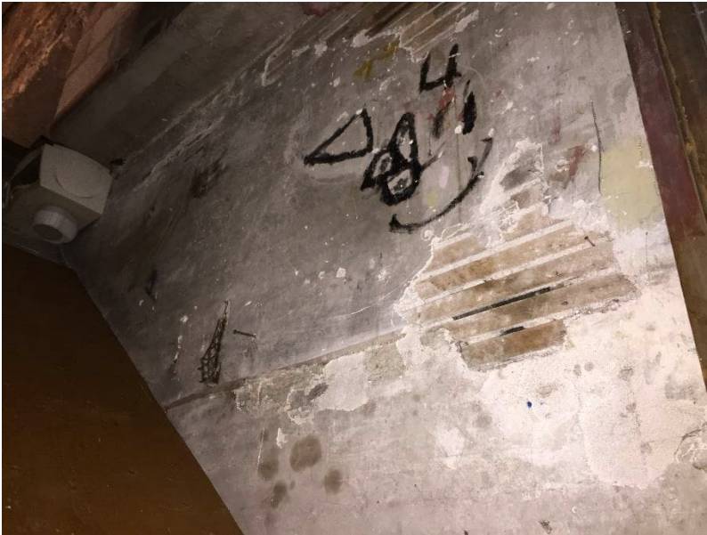
Photo 6: View of asbestos-containing wall plaster observed to be in poor condition in the stairwell to the basement of the subject building.
