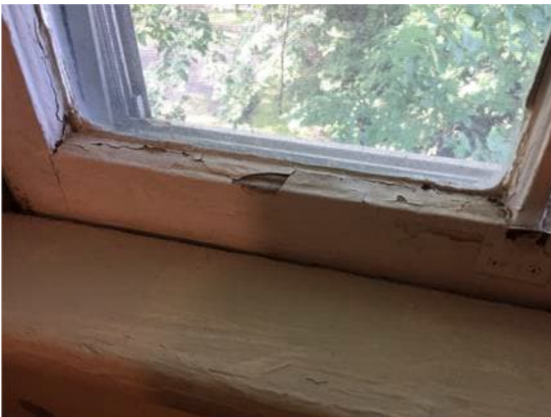
Photo 7: View of lead-containing white paint observed to be in poor condition in Room E on the 2 nd floor of the subject building.
