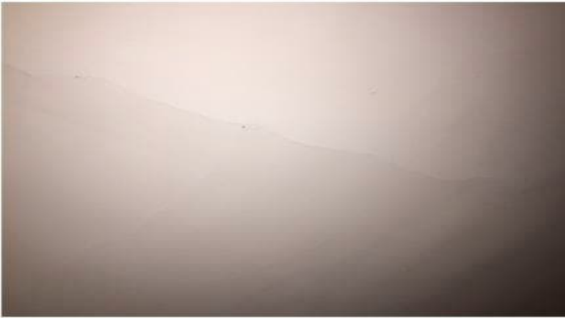
Photo 4: View of asbestos-containing ceiling plaster observed to be in fair condition in Room B on the 1 st floor of the subject building.
