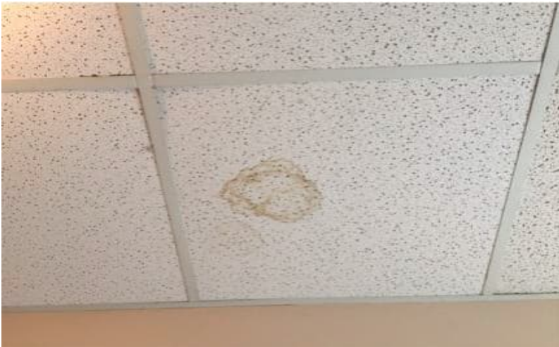
Photo 8: View of water-damaged ceiling tile observed in the living room on the 1 st floor of the subject building,
