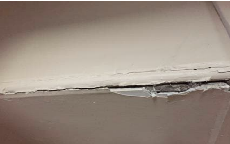
Photo 5: View of asbestos-containing ceiling plaster observed in poor condition in the hallway on the 2 nd floor of the subject building
