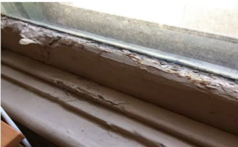
Photo 6: View of lead-containing beige paint observed to be in fair condition in Room A on the 2 nd floor of the subject building.
