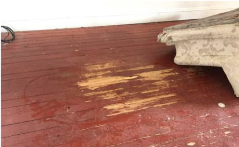
Photo 7: View of lead-containing maroon paint observed to be in poor condition in Room B on the 3 rd floor of the subject building.
