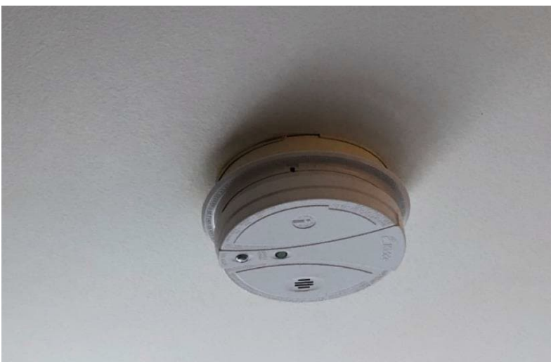
Photo 9: Typical view of smoke detectors containing radioactive materials.
