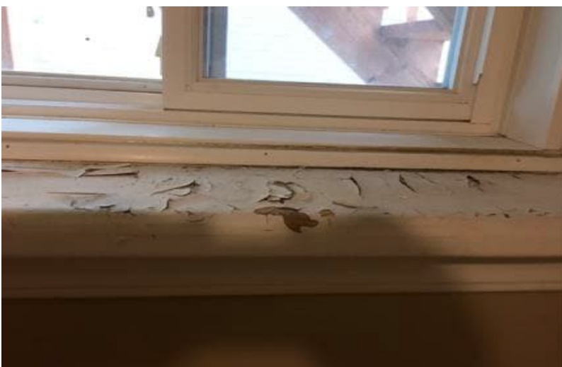
Photo 6: View of lead-containing white paint observed to be in poor condition in bathroom of the first floor.
