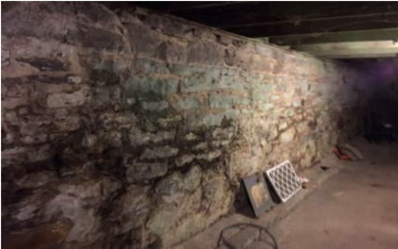
Photo 4: View of typical finishes observed at the building located at 118 Henderson Avenue.
