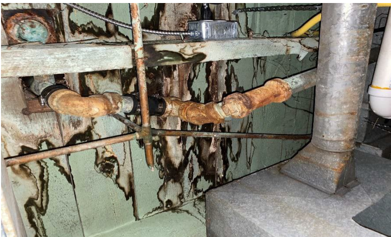
Photo 8: View of water damage and growth observed on the ceiling in the basement.
