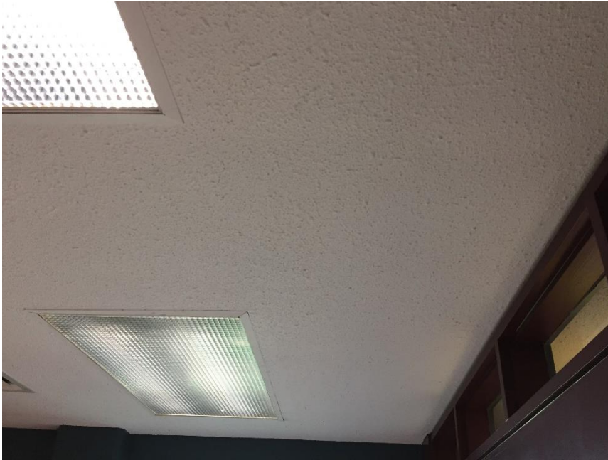
Photo 3: View of asbestos containing texture coat (popcorn ceiling) in Room 172.
