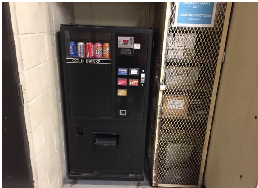
Photo 8 View of vending machine suspected to contain ODS in Room 100C
