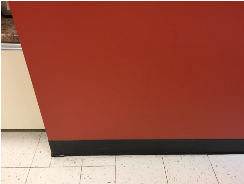
Photo 4: View of red lead containing paint in Room 179
