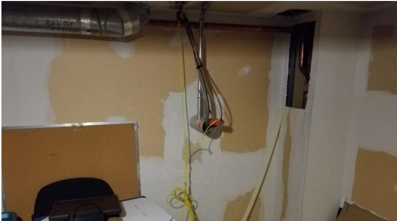
Photo 1: A typical view of an asbestos-containing drywall joint compound was observed throughout the subject building.
