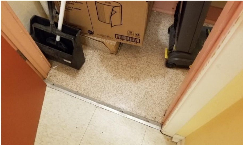
Photo 4: View of non-asbestos Vinyl Sheet Flooring (Grey and White) and non-asbestos 12"x12" vinyl floor tiles (White w/ Grey Flakes).
