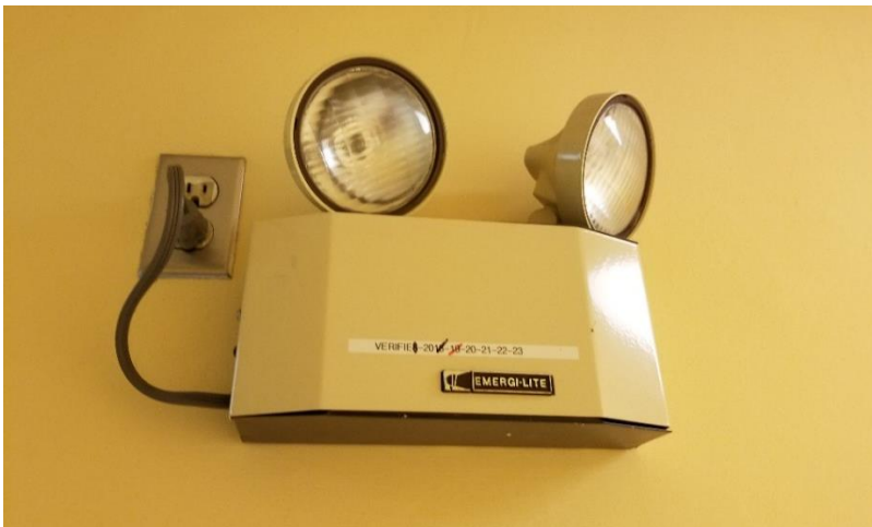
Photo 5: A typical view of lead-battery packs was observed throughout the subject building.
