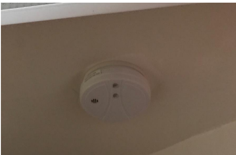
Photo 6: A view of the radioactive-containing smoke detector was observed throughout Room 300.
