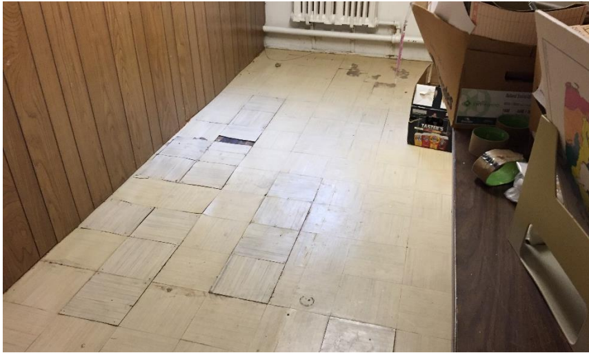
Photo 4: View of the asbestos-containing vinyl floor tiles (12"x12" – Beige w/ Brown Lines) observed throughout the basement level.
