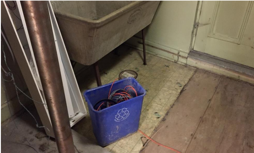
Photo 7: View of the asbestos-containing vinyl sheet flooring (Yellow Rectangular Pattern) observed in Room B9.
