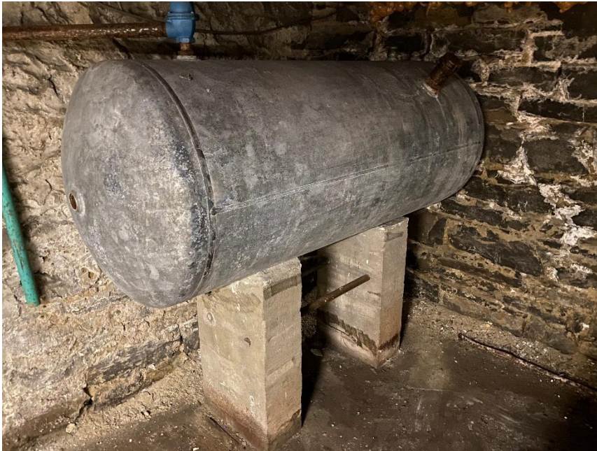
Photo 3: View of the removed asbestos-containing boiler tank insulation (paring cement) observed to have been abated from Room B5.
