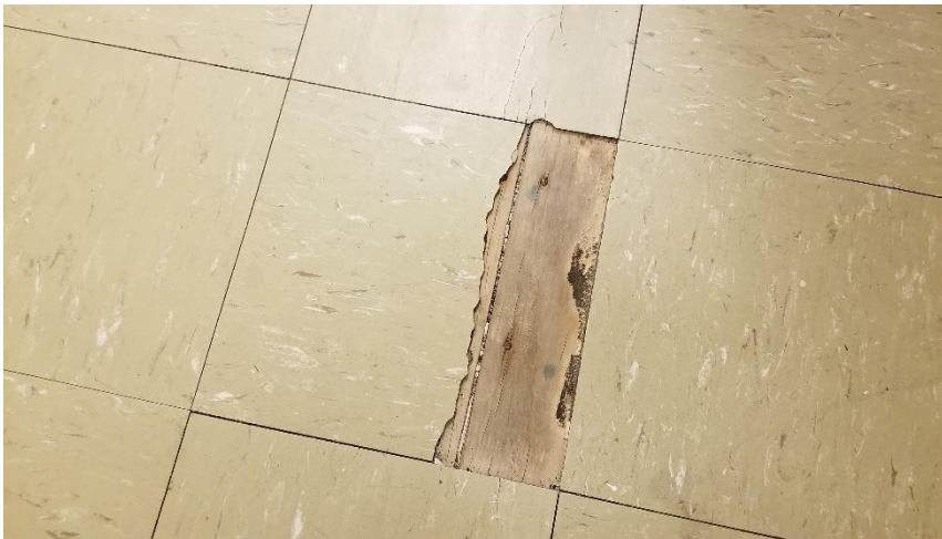
Photo 11: Representative view of the asbestos-containing vinyl floor tiles (12"x12" – Green) observed in poor condition in Room 101.
