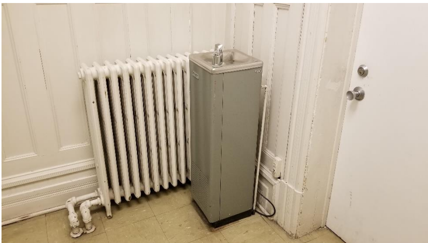
Photo 9: Representative view of equipment observed to contain ODSs in Room 101.
