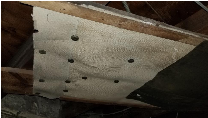
Photo 4: View of the asbestos-containing paper insulation (Grey) observed in poor condition in Room B5.
