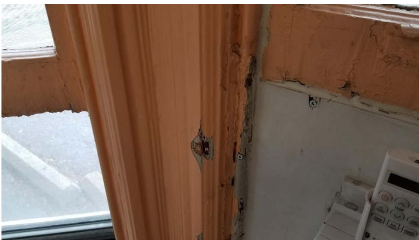
Photo 17: View of the lead-containing frame paint (Peach) observed in poor condition in Room 108.
