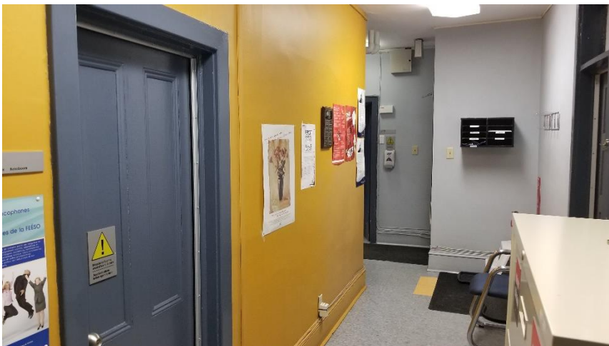
Photo 20: Representative view of the lead-containing paint (Dark Yellow) observed in good condition throughout the second floor.
