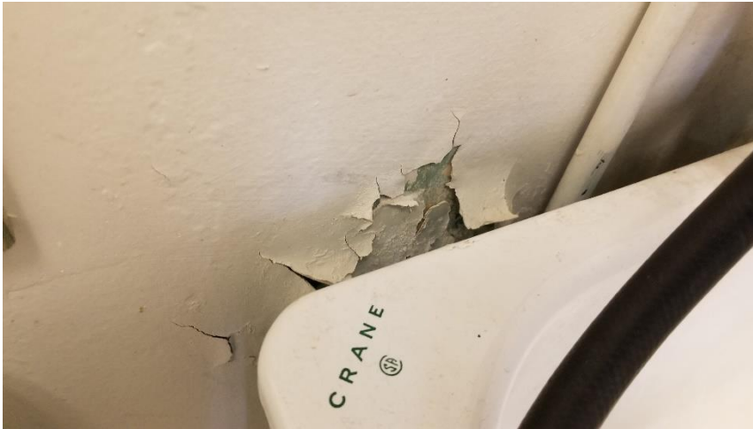
Photo 13: View of the lead-containing wall paint (White) observed in poor condition in Room 103 during the 2022 Reassessment.
