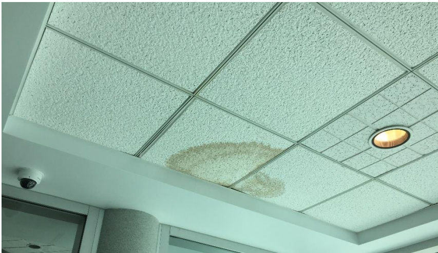
Photo 5: View of water damaged ceiling tiles observed in Room 100G.
