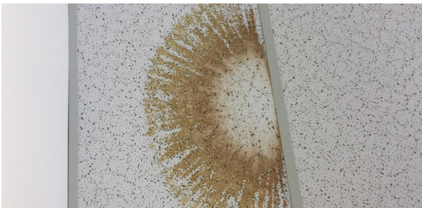
Photo 6: View of water damaged ceiling tiles observed in Room 100G.
