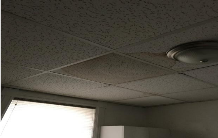
Photo 1: View of water damaged ceiling tiles (2'x2') observed in the kitchen within the subject building.
