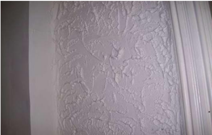
Photo 2: View of the non-asbestos-containing texture coat observed in the front room on the 1 st floor of the subject building.
