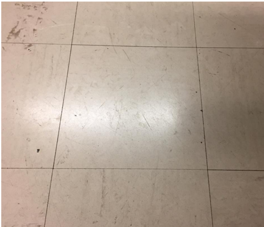
Photo 2: View of asbestos-containing vinyl floor tiles observed in Room M12 of Subject Building.
