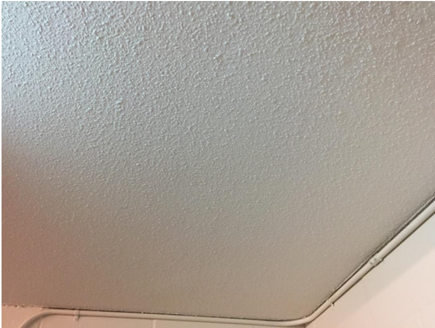
Photo 1: View of asbestos-containing textured ceiling observed in Room M03, M10, M11, and M12 of Subject Building.
