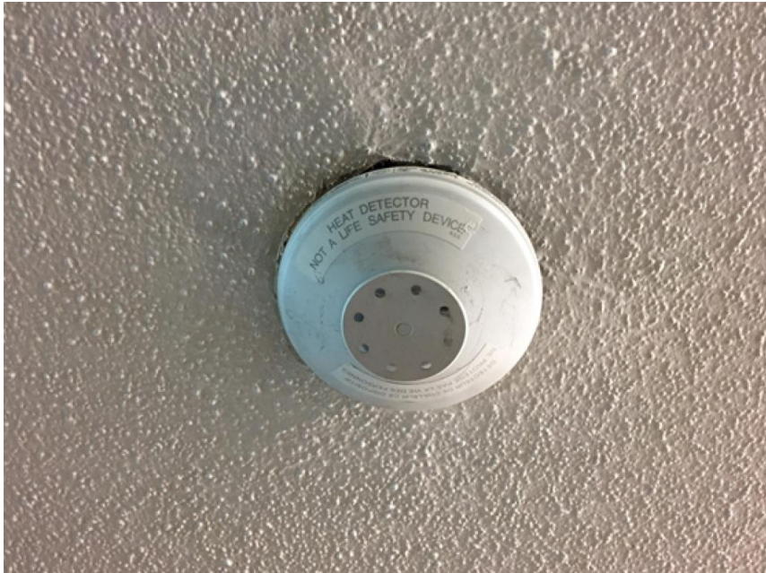
Photo 5: View of Radioactive Smoke Detector observed in Room M03 of Subject Building.
