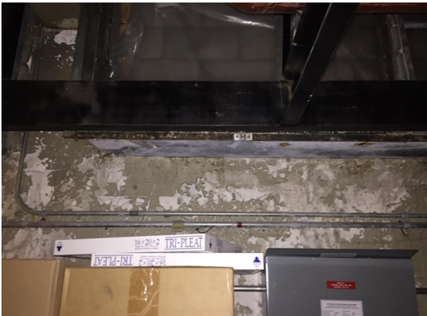
Photo 4: View poor condition grey wall paint observed in Room M09. Sample PB6
