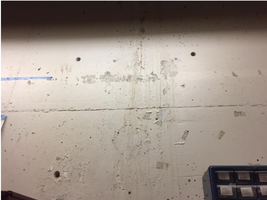
Photo 3: View of poor condition white wall paint observed in Room M13. Sample PB1
