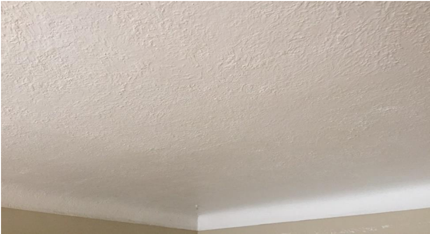
Photo 4: View of previously identified asbestos-containing ceiling texture coat observed in Room 103.
