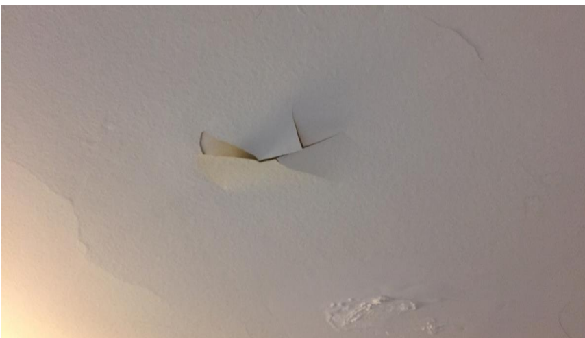
Photo 6: View of damaged low levels of lead white paint observed on the ceiling of Room 101.
