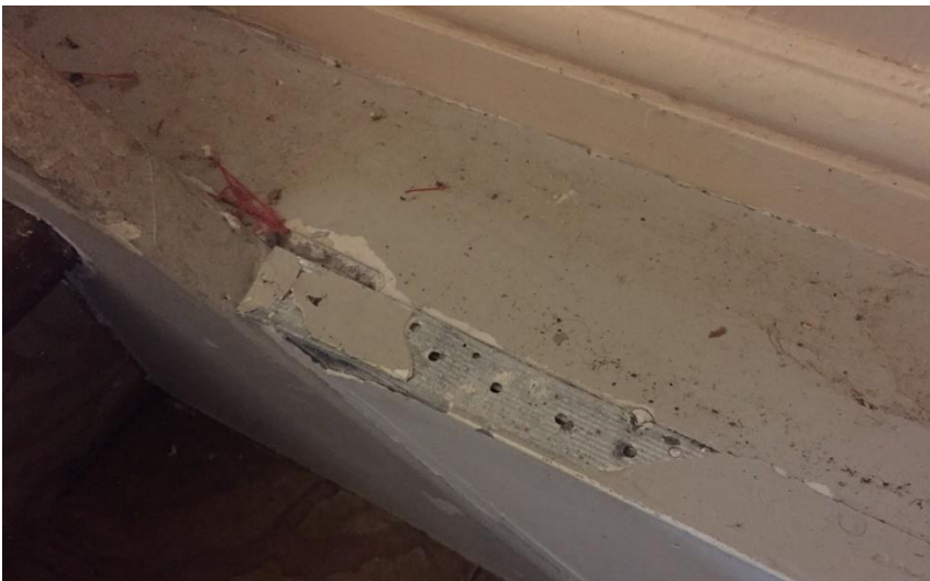
Photo 5: View of damaged asbestos-containing drywall joint compound observed in Room 00.
