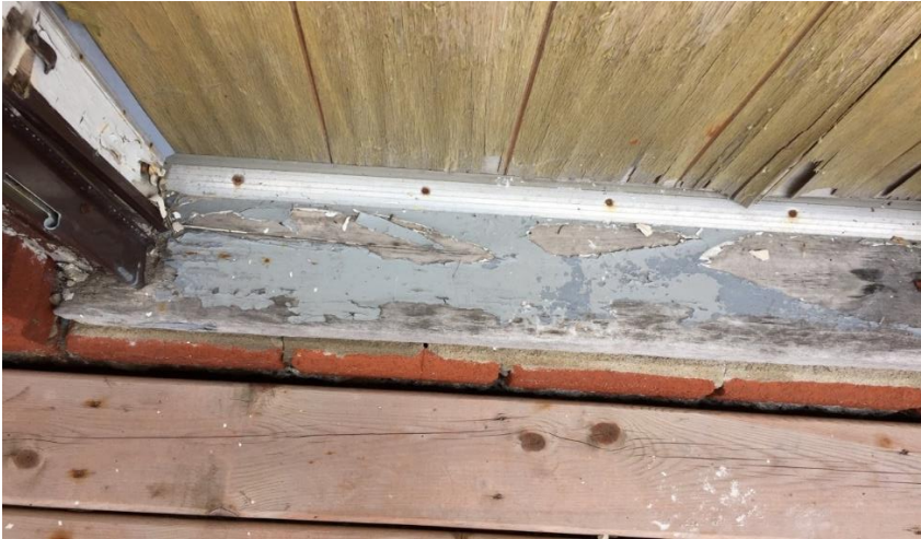
Photo 7: View of damaged lead-containing grey paint observed on the exterior front porch.
