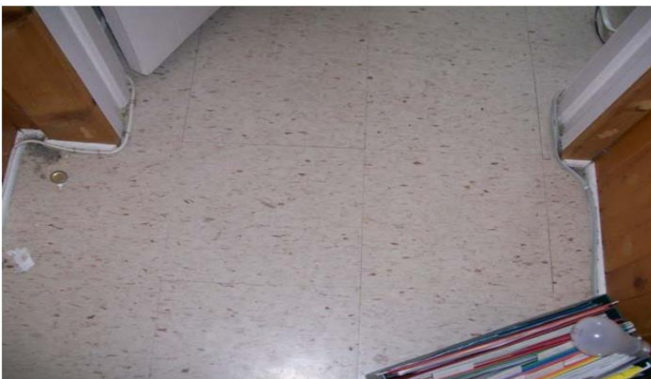
Photo 3: A view of non-asbestos-containing vinyl floor tile was observed in the kitchen on the 1 st floor of the subject building.
