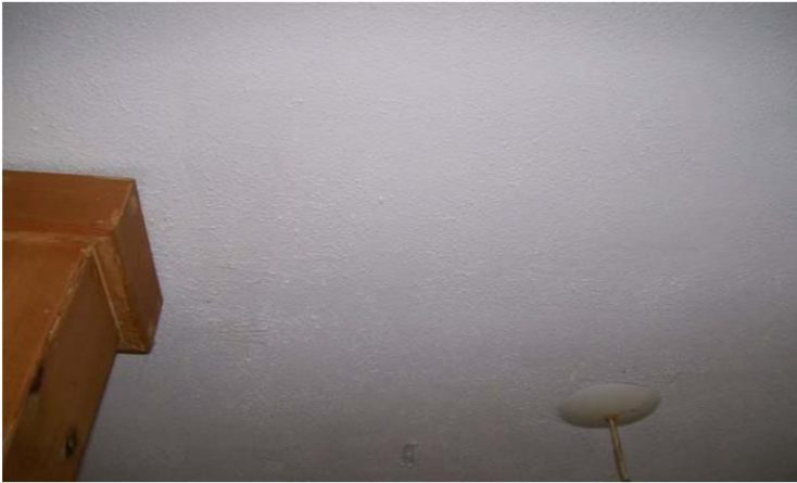
Photo 1: A view of asbestos-containing texture coat observed in the main room on the 1 st floor of the subject building.
