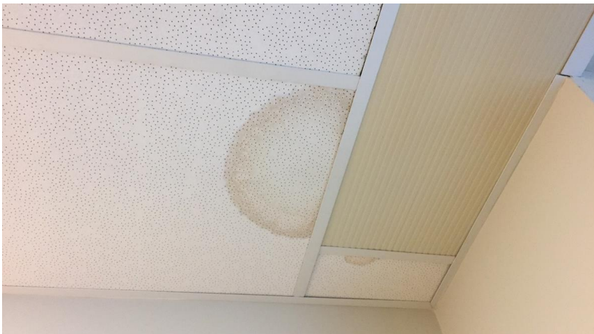
Photo 11: Representative view of the water damaged ceiling tiles observed in select areas of the subject building.
