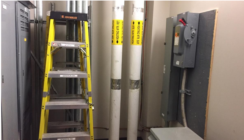
Photo 4: Representative view of the non-asbestos containing mechanical insulation observed throughout the subject building.
