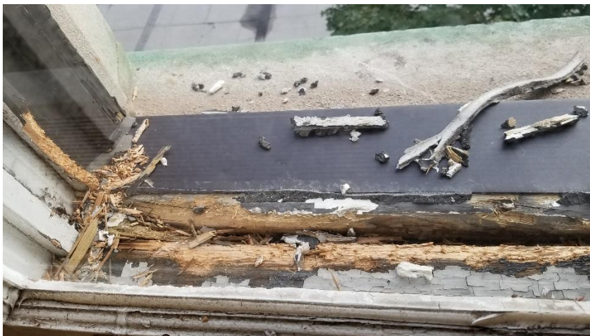
Photo 14: View of the poor condition lead window frame paint (White) observed in Room 302.
