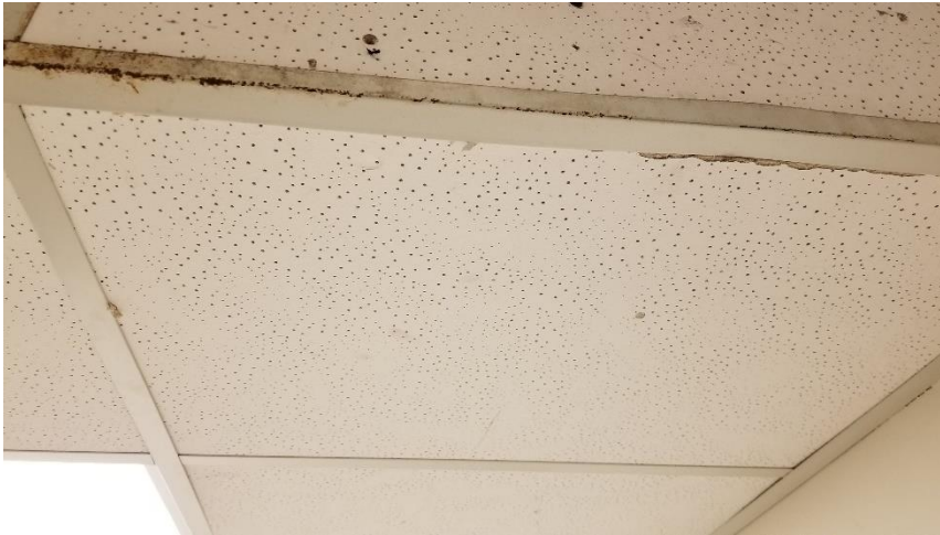
Photo 16: View of the asbestos-containing ceiling tiles (2'x4' White w/ Small Pinholes) observed in Room 106.
