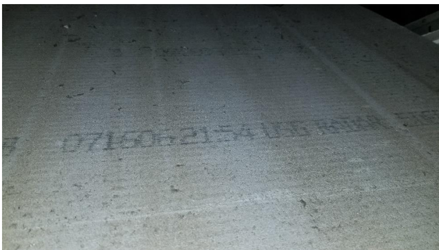
Photo 15: View of the date stamped suspended ceiling tiles (2'x4' – Pinholes & Small Fissures) observed throughout the subject building.
