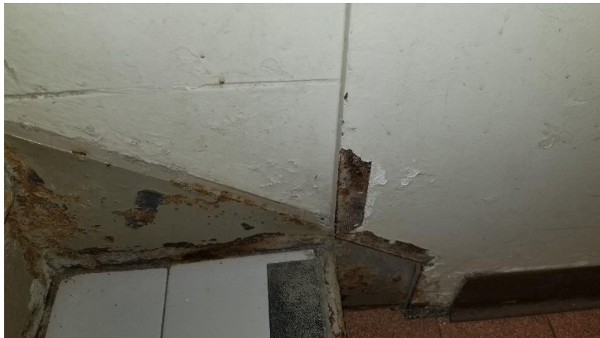
Photo 7: View of the poor condition asbestos-containing drywall joint compound observed in Room 106.
