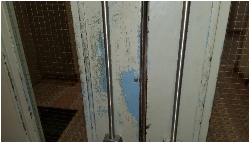
Photo 5: View of the poor condition lead paint (Blue) observed on the doors of Room 106.
