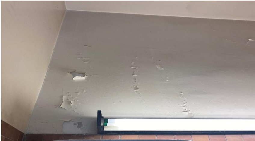
Photo 4: View of the water damaged ceiling and wall paint identified in Room 101A.
