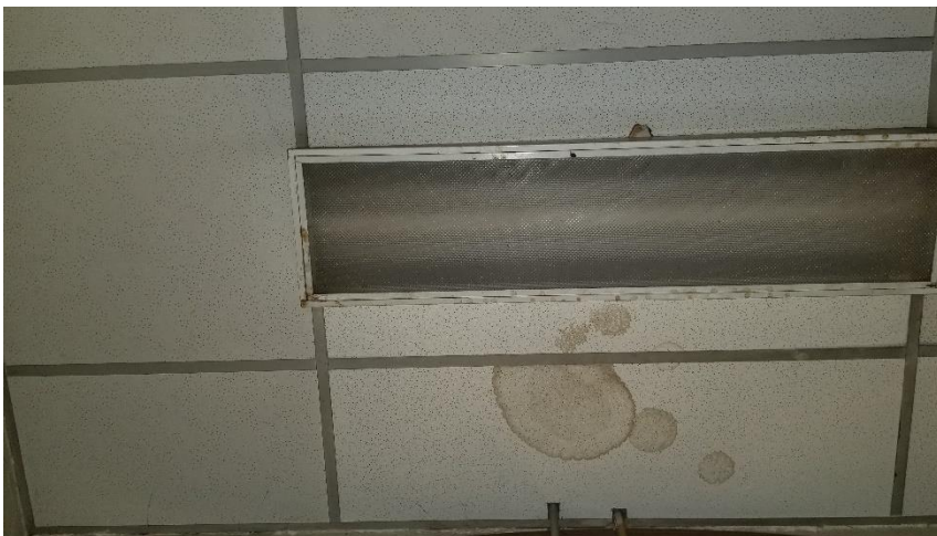
Photo 6: View of the water damaged ceiling tiles identified in Room 106A.
