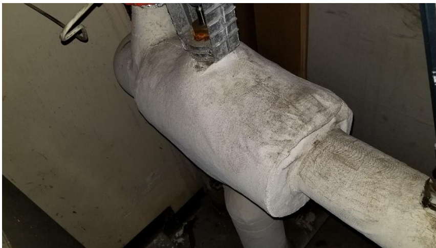
Photo 12: View of the fiberglass mechanical pipe fitting and pipe straight insulation observed throughout the subject building.
