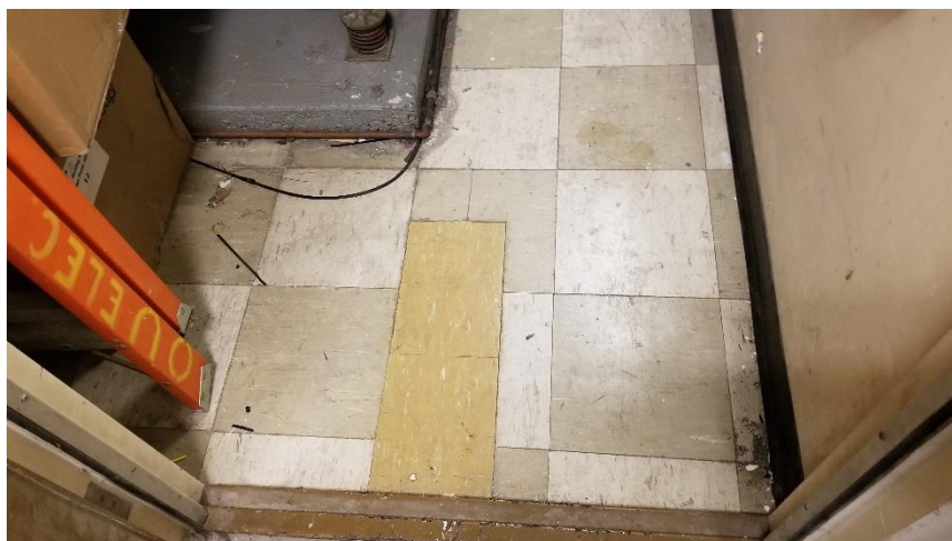
Photo 9: View of the asbestos-containing vinyl floor tiles: (12"x12" – Gold w/ White Streaking), (12"x12" – Grey w/ Streaks), and (12"x12" – Beige w/ Streaks) observed in Room 107J.
