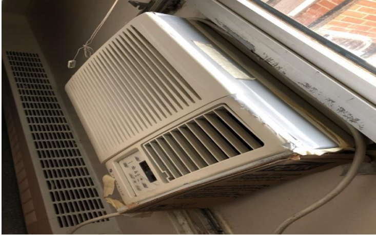
Photo 12: Typical view of ODS containing air-conditioning unit.
