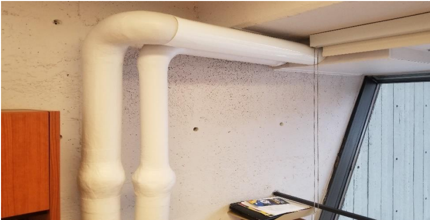
Photo 1: View of asbestos-containing pipe fitting insulation observed in Room 306B.
