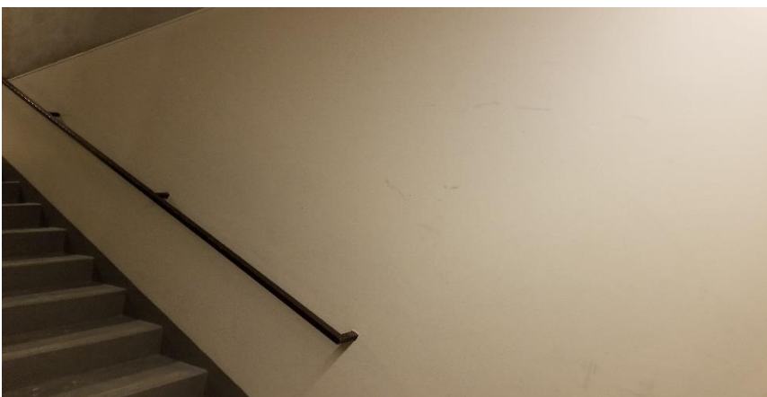
Photo 3: Typical view of asbestos-containing drywall observed throughout the subject building.
