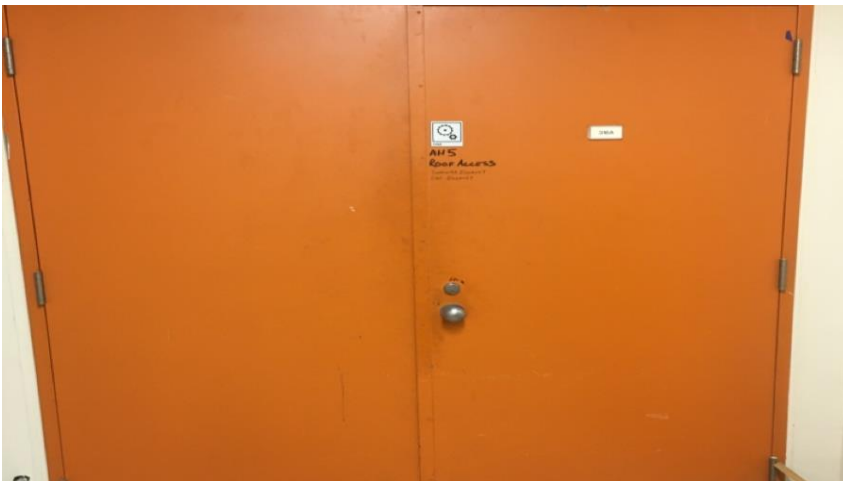
Photo 7: View of orange lead-containing paint observed on the door of Room 316.
