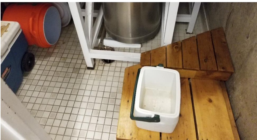
Photo 11: View of ceramic floor tiles grout observed throughout the subject building suspect to contain asbestos.
