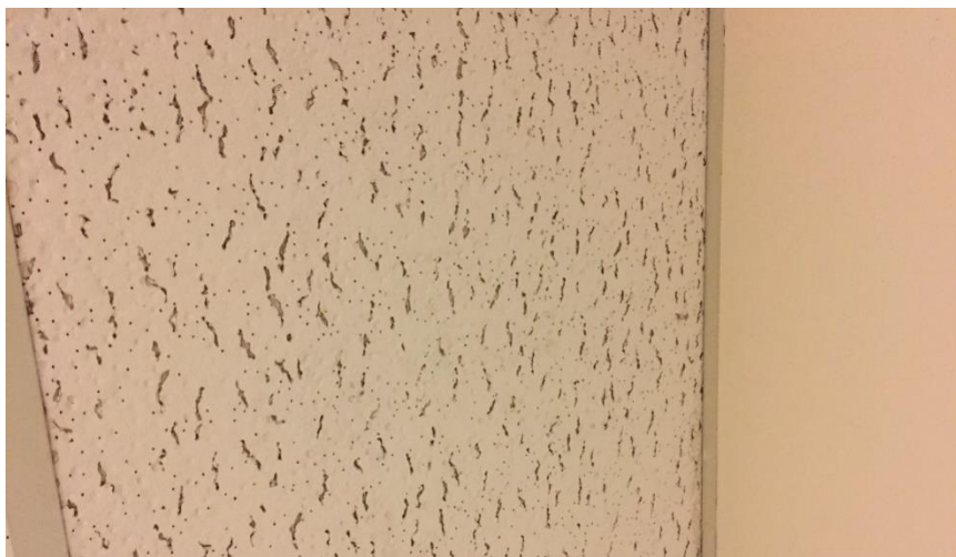
Photo 4: View of asbestos-containing suspended ceiling tiles observed in Room 415.
