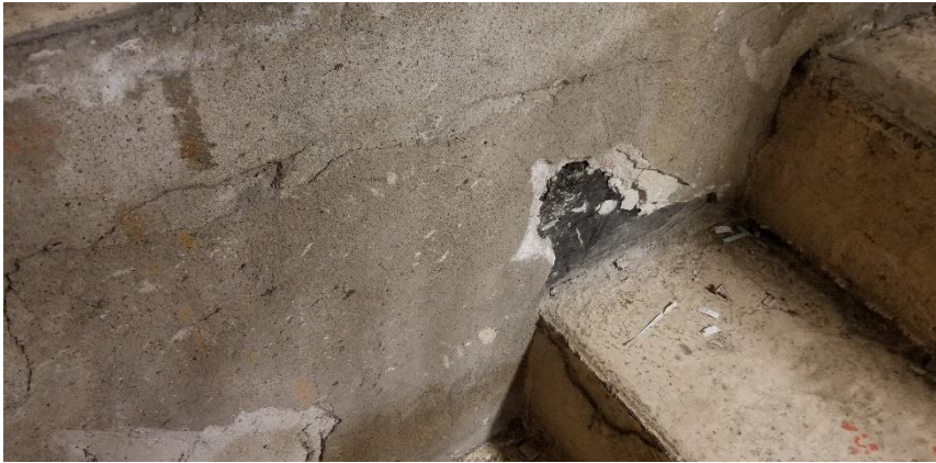
Photo 7: View of asbestos-containing wall plaster observed to be in poor condition in Room 0189.
