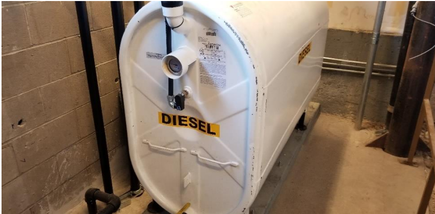
Photo 10: View above ground storage tank observed to be in good condition in Room 7028A.
