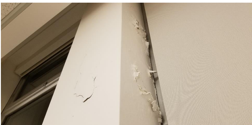
Photo 6: View of asbestos-containing wall plaster observed to be in poor condition Room 1076.
