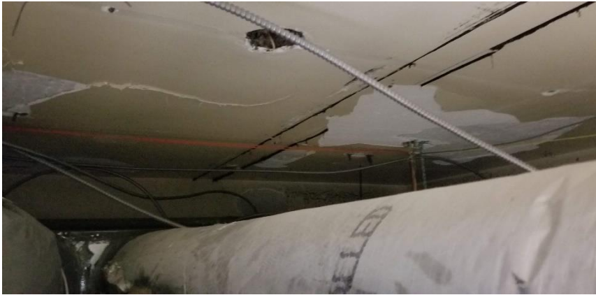
Photo 1: View of asbestos-containing tar (Black) observed to be in fair condition on the plaster ceiling in Room 1021.
