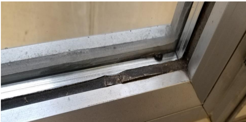
Photo 2: View of asbestos-containing window caulking observed to be in good condition in Room 1070 and other stairwells throughout the subject building.
