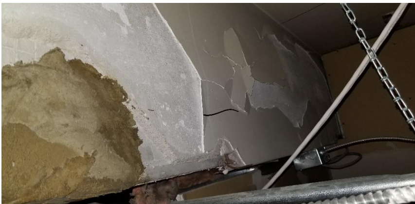
Photo 3: View of asbestos-containing wall plaster observed to be in poor condition in Room 5082.
