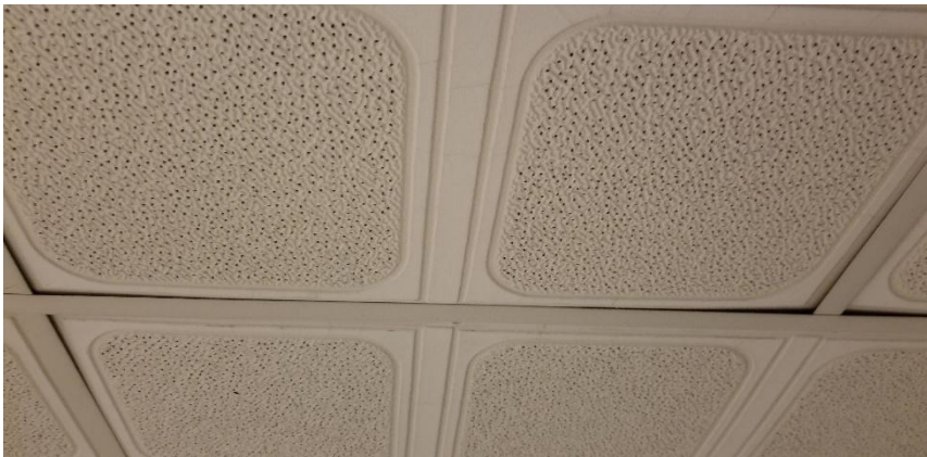
Photo 8: View of non-asbestos containing suspended ceiling tiles (2'x4'-Square Pattern with Pinholes) observed in Room C219.
