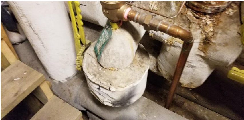
Photo 5: View of asbestos-containing mechanical pipe fitting insulation observed to be in good condition in Room C01B.
