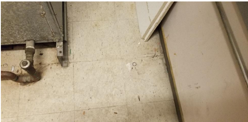
Photo 9: View of non-asbestos containing vinyl floor tiles (12"x12"-Off White with Small Grey Streaks) observed in Room N0122B.
