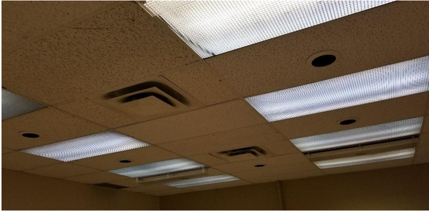
Photo 10: View of asbestos-containing suspended ceiling tiles (2'x4"-White Tone) observed to be in good condition in Room C012A.
