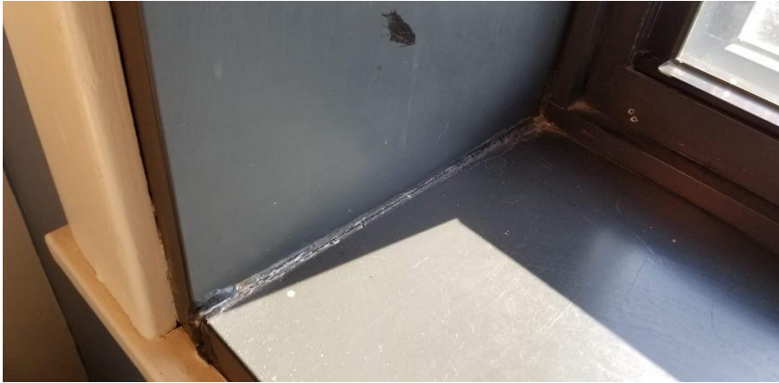
Photo 7: View of asbestos-containing window frame caulking observed to be in fair condition in Room M386F.
