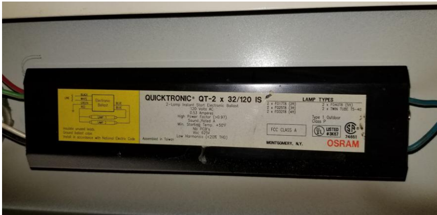
Photo 12: View of non-PCB Containing light ballasts observed in C459.
