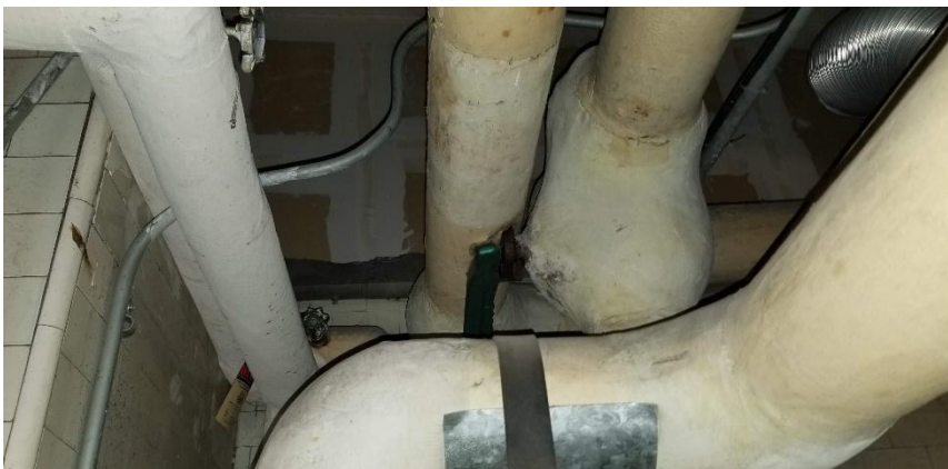
Photo 6: View of asbestos-containing mechanical pipe fitting insulation observed to be in good condition in Room C01D.
