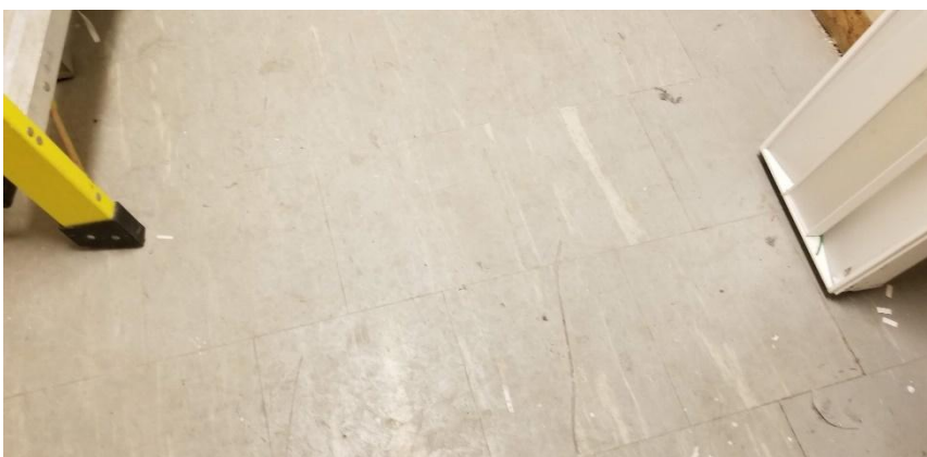
Photo 3: View of asbestos-containing vinyl floor tiles (9"x9"-Grey Coloured) observed to be in good condition in Room C08.
