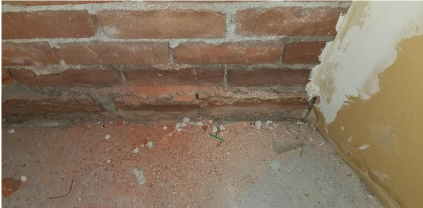
Photo 4: View of the asbestos-containing brick mortar observed to be in poor condition in Room C455.
