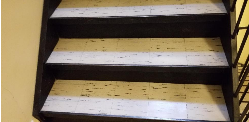
Photo 1: View of asbestos-containing vinyl floor tiles (9"x9"-White and Black) observed to be in good condition in C207C.
