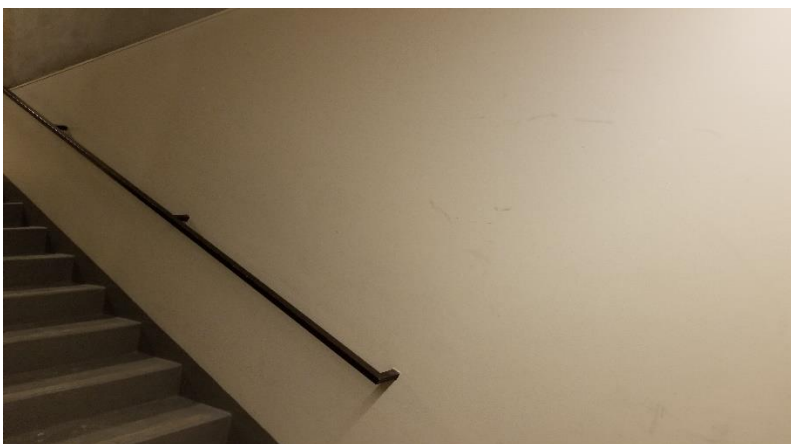
Photo 3: Typical view of asbestos-containing drywall observed throughout the subject building.
