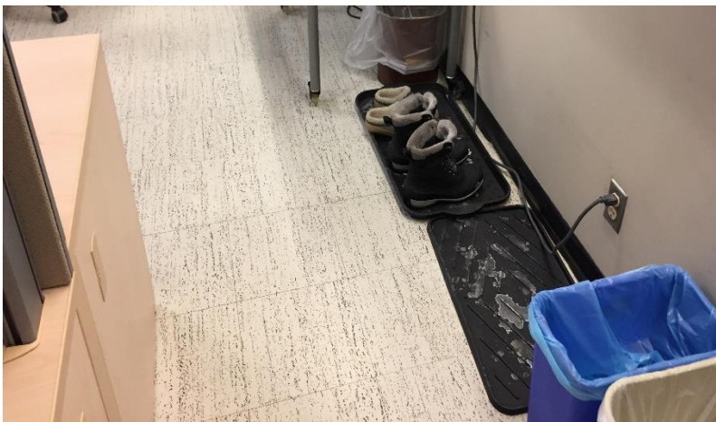
Photo 2: View of asbestos-containing vinyl floor tiles observed in Room 428.
