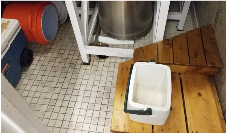
Photo 11: View of ceramic floor tiles grout observed throughout the subject building suspect to contain asbestos.
