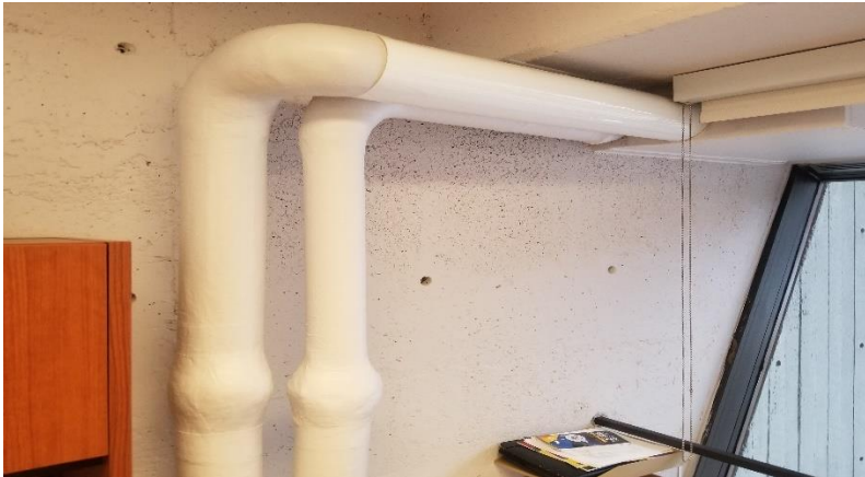
Photo 1: View of asbestos-containing pipe fitting insulation observed in Room 306B.
