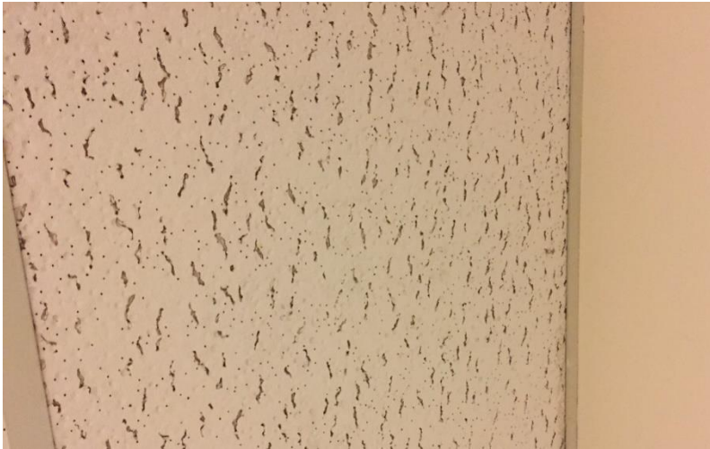
Photo 4: View of asbestos-containing suspended ceiling tiles observed in Room 415.
