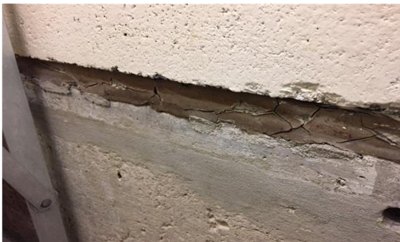
Photo 5: View of asbestos-containing wall caulking (tan) observed in Room 0024 observed to be in fair condition.
