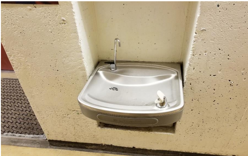
Photo 12: Typical view ODS containing water fountains observed throughout the subject building.
