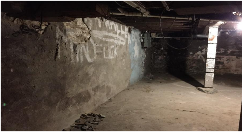
Photo 5: View of asbestos-containing texture coat observed to be in poor condition in the basement.
