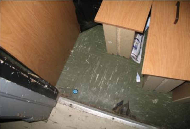
Photo 4: View of previously sampled asbestos-containing vinyl floor tile in the southside bedroom, now presumed to be under new flooring. (Ref. 0459870 (27))
