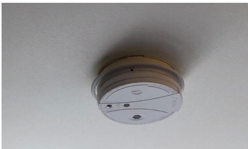
Photo 9: Typical view of smoke detectors containing radioactive materials.
