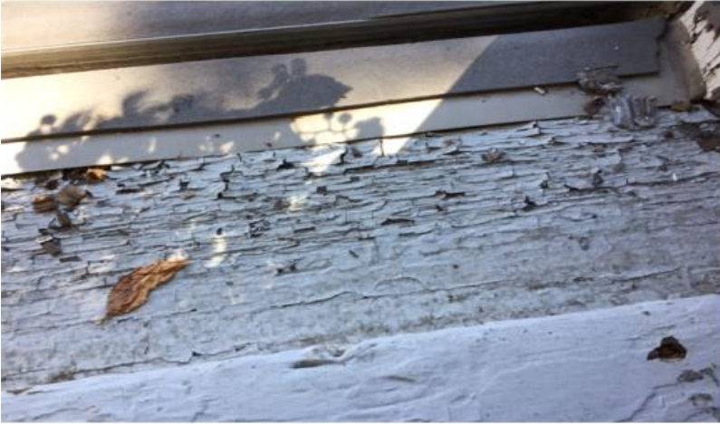
Photo 6: View of lead-containing white paint observed to be in poor condition in Room E on the 2 nd floor.
