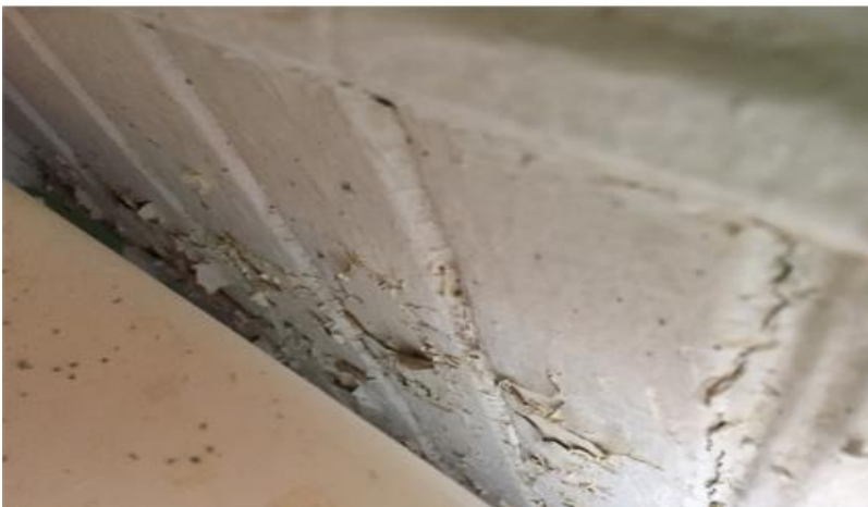
Photo 5: View of lead-containing white paint observed to be in poor condition in the bathroom on the 2 nd floor.
