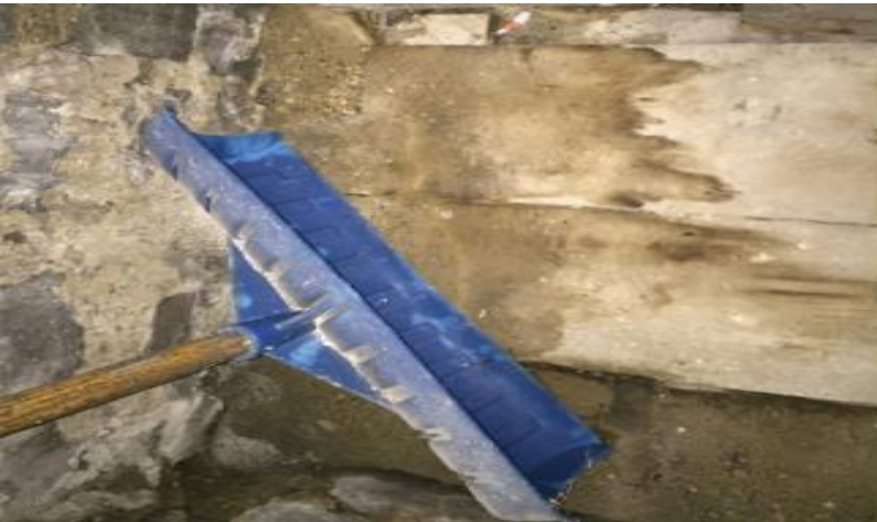
Photo 7: View of water-damaged wood stairs in the basement.
