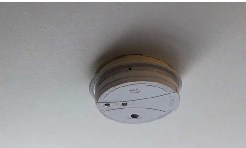
Photo 8: Typical view of smoke detectors containing radioactive materials.
